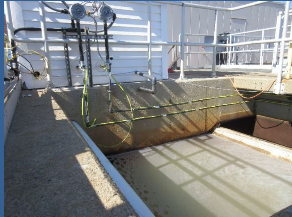
Chlorine Contact Tanks
