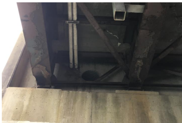
Figure 2. Abutment penetration at east abutment of I-95 bridge.
