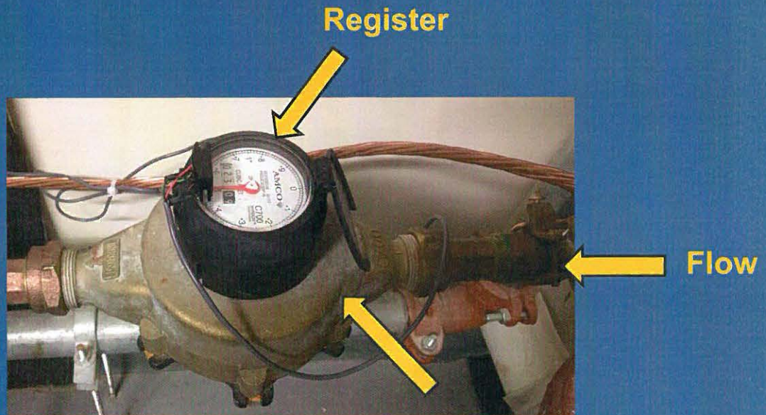
Water Meter (5/8-Inch Meter)
