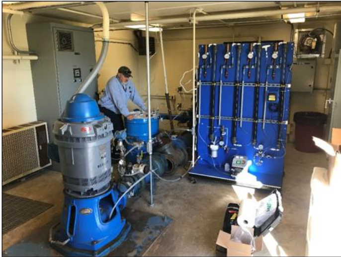
Haven Well Pump
