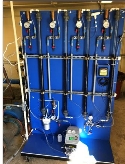
Pilot Treatment System
