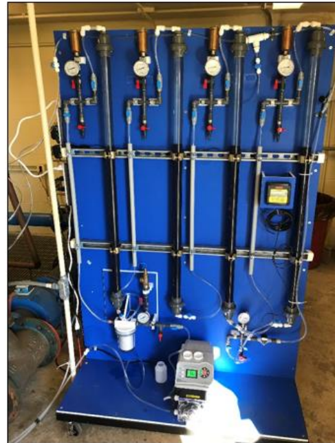
Pilot Treatment System
