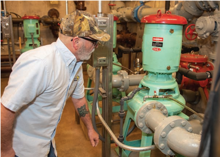
Dale Youngers, shown with the Smith & Loveless pump that transfers inflow to the biological nutrient removal system, believes in close communication with village trustees.
