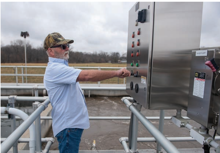
Youngers is shown at the electrical control panel for the plant’s two submersible mixers (Wilo USA).
