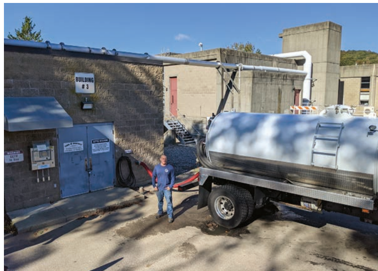
Operator Scott Farrington with the Septage Acceptance Plant at the Montville clean-water facility.
