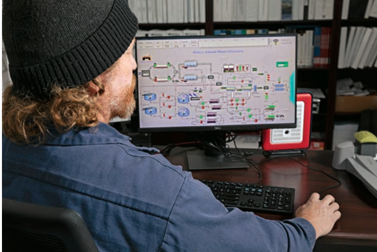
An iFIX SCADA system (GE Digital), being operated here by operator Kevin Daley, helps the plant team keep tabs on equipment and the process.
