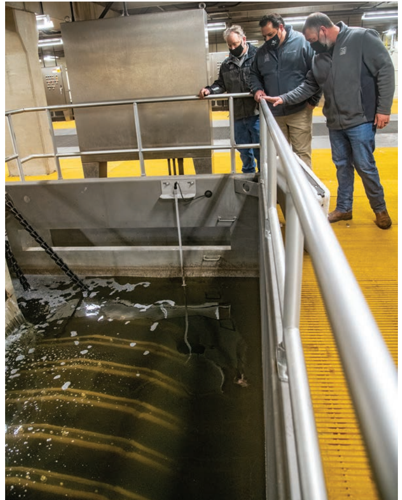
From left, Layne DelValley, Lagle and Justin Profancik survey the cloth media tertiary filters (Aqua-Aerobic Systems).
