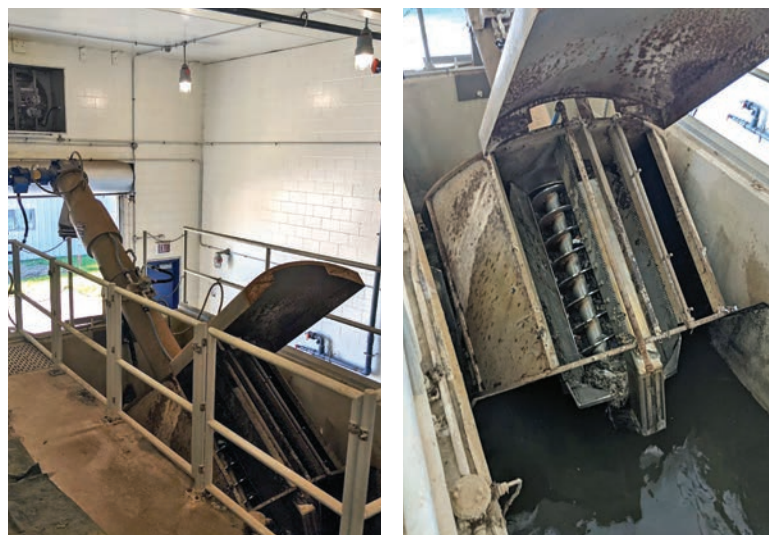
The fine screen’s angled installation and screen bars of varied heights maximize removal efficiency and minimize headloss. It also effectively removes debris such as rags and plastics.
