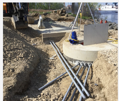
SANITARY PUMP STATION NO. 2
