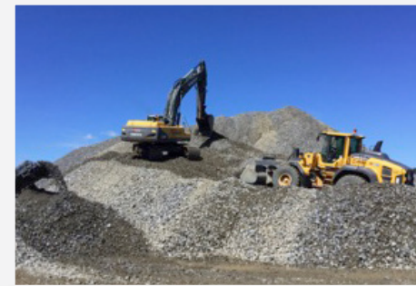
EXCAVATED STONE CRUSHED OVER 8,000 CUBIC YARDS (ABOUT TWO OLYMPIC SIZE POOLS) OF ROCK WAS REMOVED FOR EXCAVATION OF THE BIOLOGICAL AERATED FILTER (BAF). MOST OF THIS MATERIAL WAS CRUSHED AND WILL BE RE-USED ON SITE, REDUCING TRUCK TRAFFIC.
