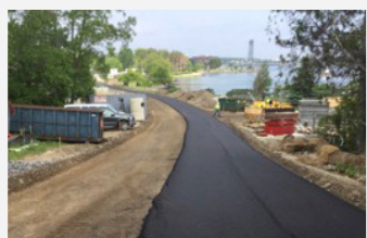
PAVED ACCESS ROAD TO PLANT NEW WATER MAIN, PRIMARY ELECTRICAL SERVICE, AND COMMUNICATION DUCT BANKS WERE INSTALLED BENEATH THE ROAD.
