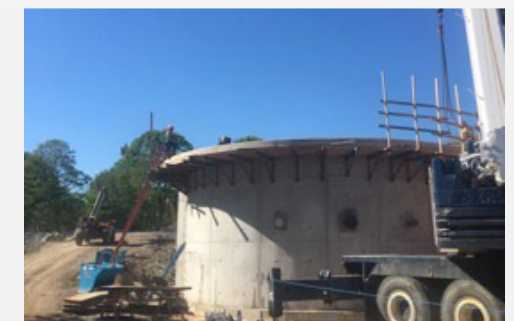
GRAVITY THICKENER NO. 2 GT2 WILL BE USED TEMPORARILY TO HOUSE SLUDGE PUMPS SO THE EXISTING ADMINISTRATION BUILDING, WHERE THESE PUMPS ARE CURRENTLY LOCATED, CAN BE DEMOLISHED. THIS WAS ONE OF THE MANY PROVISIONS PUT IN PLACE TO ALLOW THE CITY TO OPERATE THE TREATMENT FACILITY DURING CONSTRUCTION.
