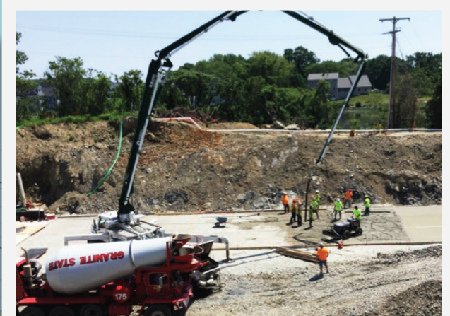
CONCRETE WORK ON BAF BLDG CONCRETE HAS TO BE PUMPED OVER AND DOWN TO THE BAF STRUCTURE WHERE THE BOTTOM IS APPROXIMATELY 25-FEET BELOW GRADE. THE CONCRETE DELIVERIES HAVE A SPECIFIC TIME FRAME THEY NEED TO MEET FROM THE TIME THEY LEAVE THE CONCRETE PLANT TO PLACEMENT IN THE CONCRETE FORMS.
