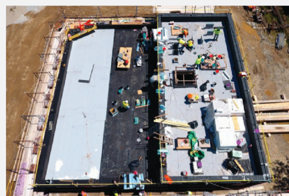
ROOFING INSTALLATION ON HEADWORKS BLDG WHITE COLORED ROOFING WAS SELECTED FOR ALL FLAT ROOFS AS A MEANS TO MINIMIZE HEAT GAIN FROM THE SUN.
