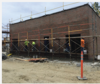
BRICK FACADE ON HEADWORKS BLDG BRICK WAS SELECTED FOR THE NEW BUILDING TO MATCH THE EXISTING FACILITIES THAT WILL REMAIN ON THE SITE. THIS FACILITY WILL BE THE MOST VISIBLE AT THE COMPLETION OF THE PROJECT AND WILL BE LOCATED JUST INSIDE THE ENTRANCE GATE.
