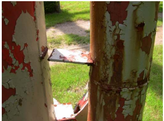
A standoff bracket at the base of the overflow pipe has broken free from the leg column.
