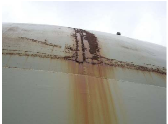
Extensive coating failure and surface corrosion extends down the knuckle plate surfaces.
