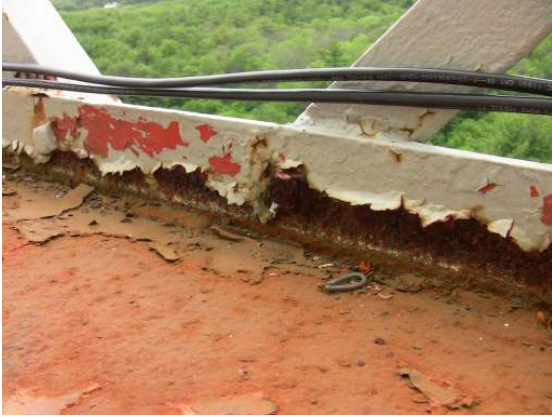
Showing coating failure and extensive corrosion resulting in some metal loss along the balcony deck and kick plate.
