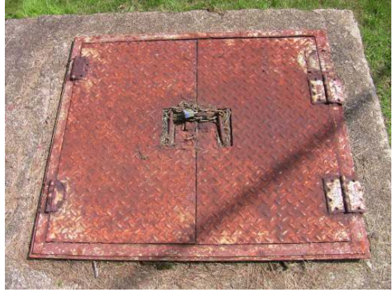
The top hatch to the valve vault is in poor condition, but was secured with a chain and lock.
