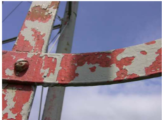
Showing extensive top coat failure and scattered corrosion along the leg column ladder cage.
