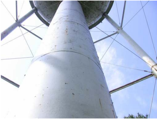
Scattered coating breakdown and corrosion along the lower riser cylinder.
