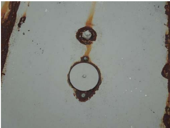
Showing an additional cathodic port and adjacent rigging plug that are in place.
