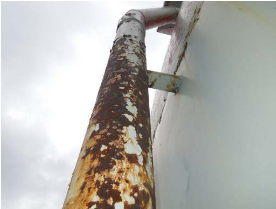
Extensive coating failure and surface corrosion along the overflow pipe surfaces adjacent to the shell.
