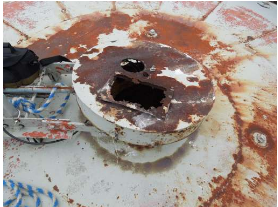
Complete failure of the existing roof finial vent will require immediate replacement.
