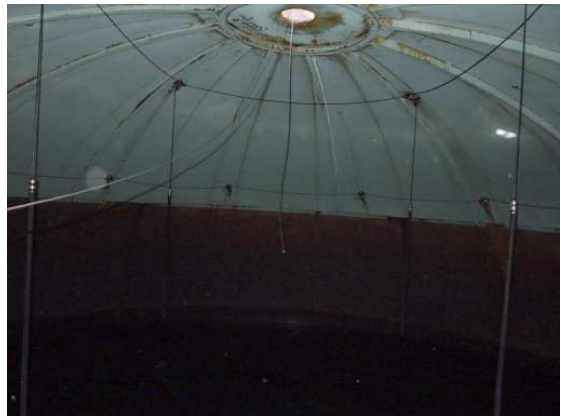
The interior roof is equipped with cabling and insulators for the cathodic protection system, but it does not appear to be functional.
