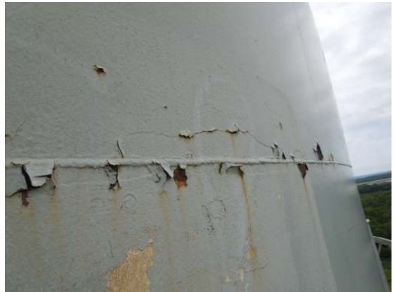
Showing areas of cracked and peeling coating along weld seams and previous spot blast profile.
