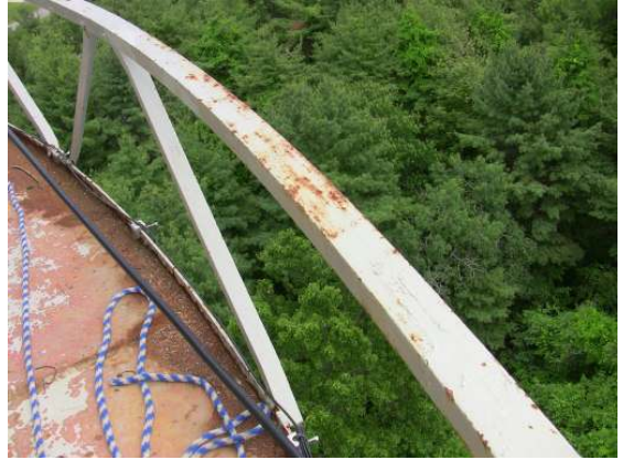
The balcony handrail measures only 32" in height and is exhibiting scattered coating failure and corrosion.
