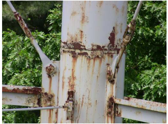
Heavy corrosion along the support column and junction points of the sway rods, radial rods and horizontal struts.
