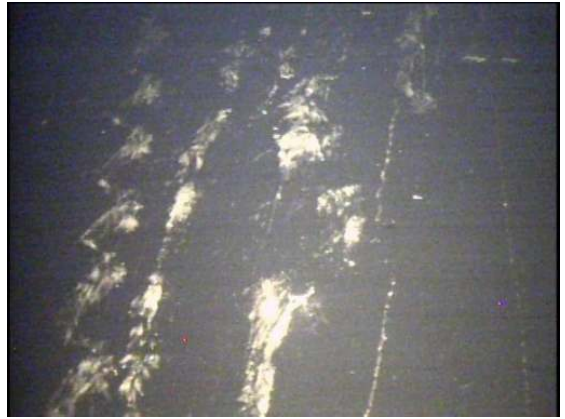
Areas of corrosion evidence through the silt layer along the lower bowl surfaces.
