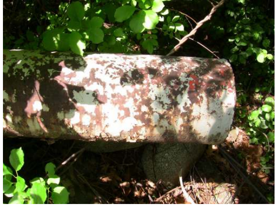
The overflow pipe terminates at the site perimeter
