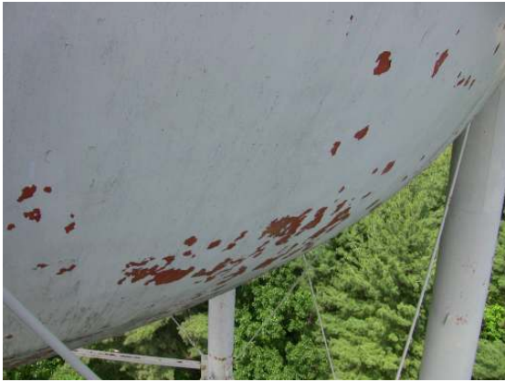
Showing widespread top coat failure along the upper bowl surfaces.
