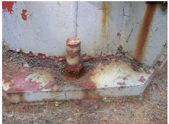
Heavy corrosion and measureable metal loss along one of the leg column anchor bolts.
