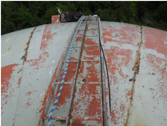
The revolving roof ladder appears to be in sound structural condition, but coatings are failing.
