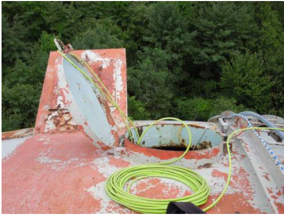
The roof is equipped with a single hatch that meets design requirements, but coatings are in poor condition.
