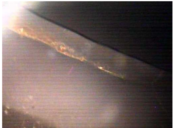
Evidence of corrosion and rust tubercle formation along the underside of the stiffener angle at the base of the knuckle.
