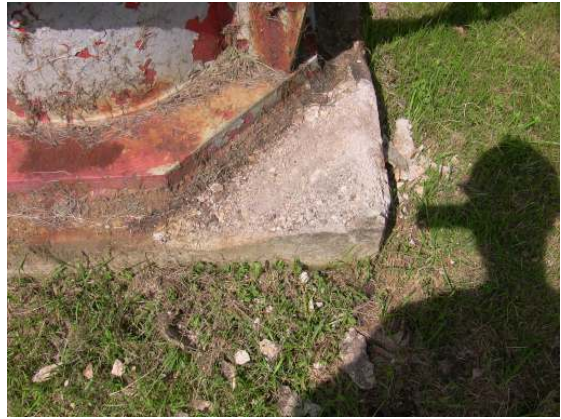
A localized area of significant surface spalling along one of the support column concrete footings.
