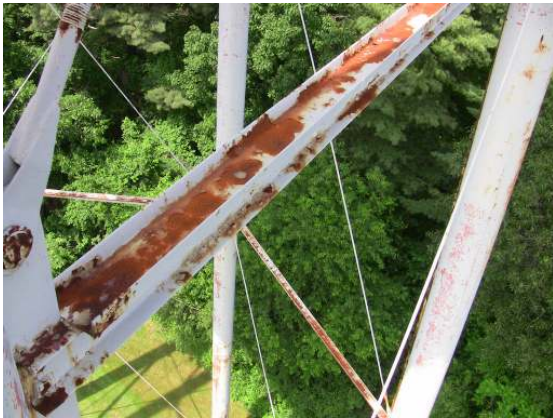
Coating failure and heavy surface corrosion along the interior channel surfaces of a horizontal strut.
