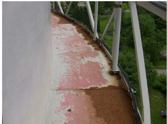
Areas of heavy corrosion along the balcony deck indicate water retention due to the lack of drainage holes.
