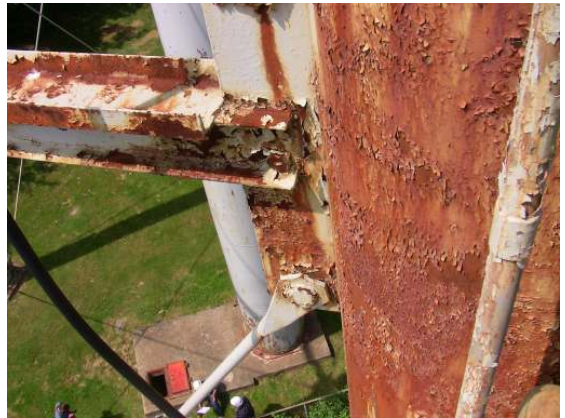
Extensive coating failure and heavy corrosion at the junction of a leg column with a horizontal strut.
