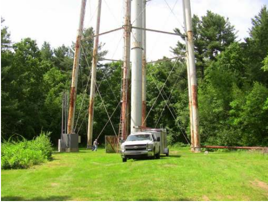
Overall view of the lower support structure surfaces indicating the extent of surface corrosion.
