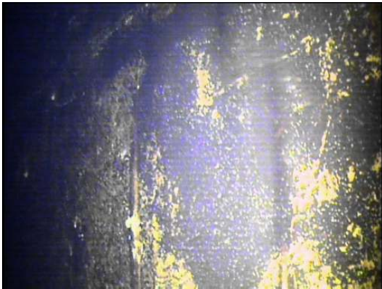
Showing widespread dense blistering throughout the shell with areas of ruptured blistering resulting in surface corrosion.
