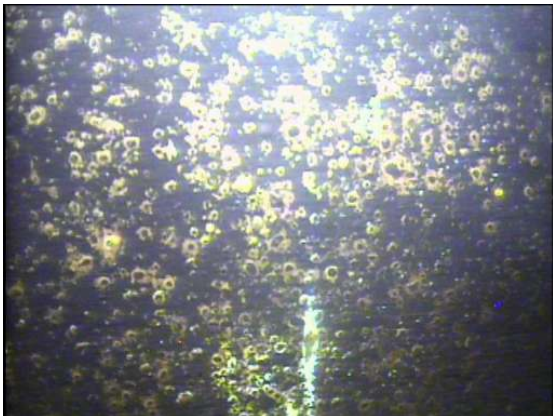
Closeup view of the dense blistering of the coating observed along the shell below water level.
