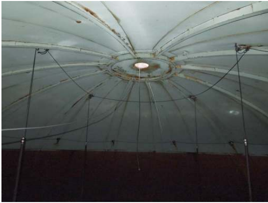
The interior roof is in fair condition, with corrosion along roof plate lap seams and the support structure.
