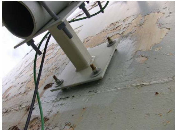
A stud welded bracket assembly secured to the shell surface is in fair to good condition.
