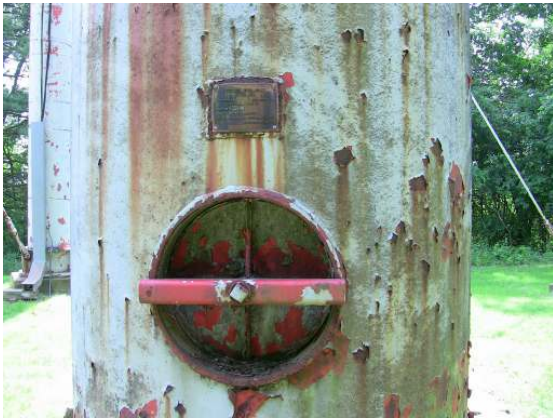
The single riser manhole is intact with no leakage, but widespread coating failure and some surface corrosion was visible.
