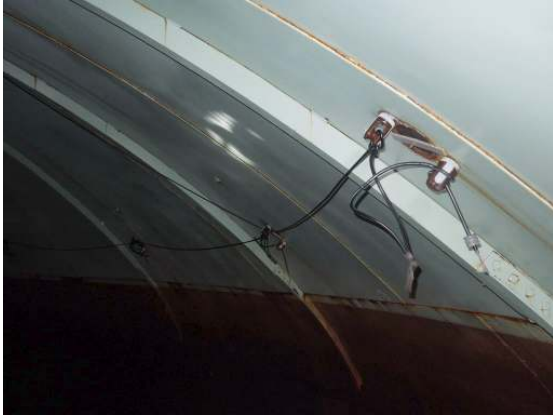
Showing disconnected components of the suspended anode cathodic protection system.
