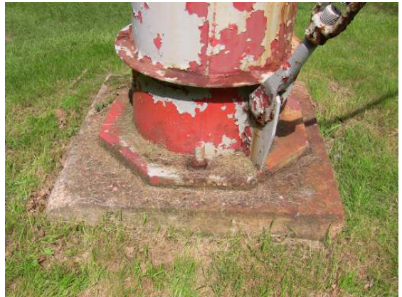
Extensive top coat failure along the base of a support column and heavy corrosion of an anchor bolt.
