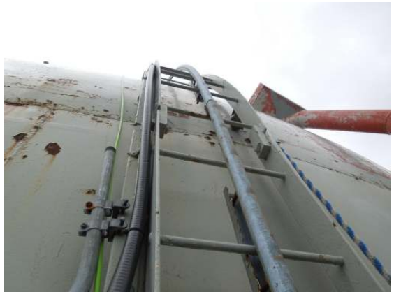
The shell segment of the access ladder is in fair condition, and is equipped with a notched rail safety climb system.
