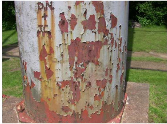
Extensive coating failure and corrosion along the bottom of the riser cylinder.
