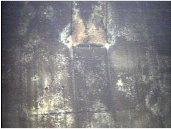
Blistering and corrosion along the upper bowl below one of the vertical shell stiffeners.
