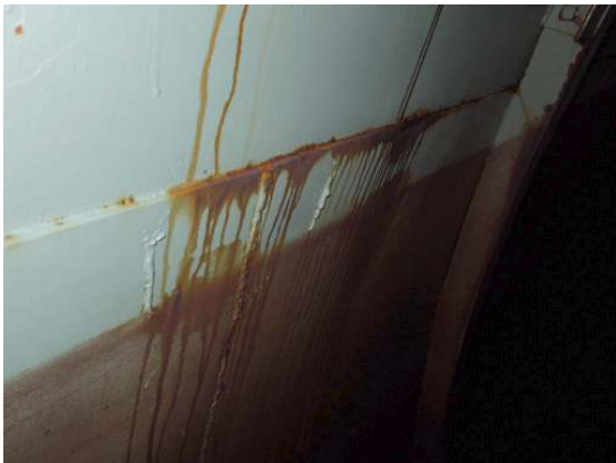
Additional areas of coating failure and surface corrosion along the roof to knuckle seam.
