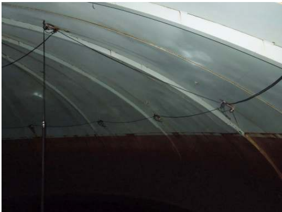
The roof plates are in generally good condition with the exception of the weld seam at the roof plate to knuckle junction.
