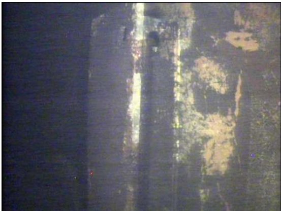
The upper portion of one of the vertical shell stiffeners showing the same coating breakdown noted throughout the shell.
