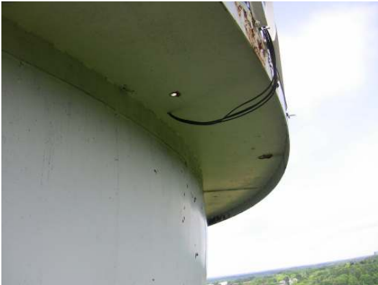
The visible underside of the balcony walkway is in fair condition, but additional coating failure was noted along the back of the kick plate.
