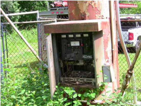
An old cathodic control unit mounted to a leg column appears to be in poor condition and non-functional.
