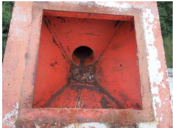
The interior coatings of the weir box are in poor condition, but the box appears to be structurally sound.
