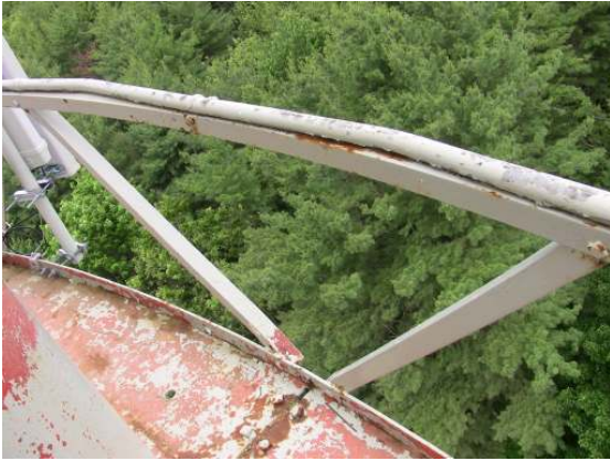
Scattered coating failure and corrosion along the balcony handrail and kick plate.
