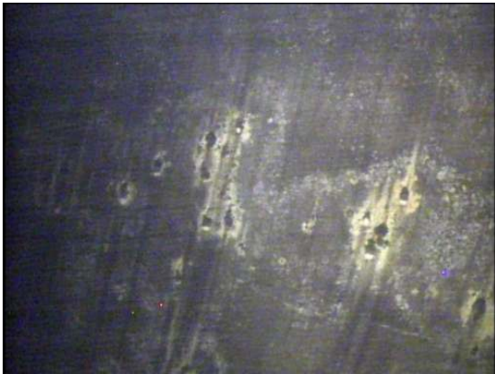
Additional areas of corrosion where breakdown of the blistered coating has occurred.
