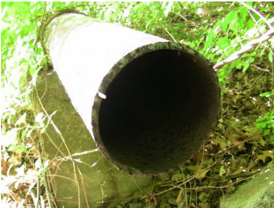
The overflow pipe discharge is not secured with a screen or flapper valve assembly.
