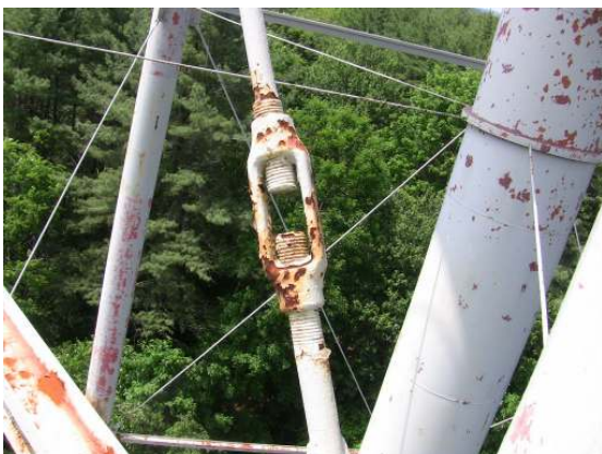
Coating failure and surface corrosion along an upper level sway rod turnbuckle.
