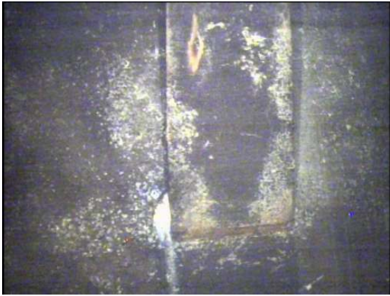
Additional blistering and coating breakdown along the lower portion of a vertical stiffener where it connects with the upper bowl.
