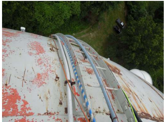
The ladder is equipped with a notched rail safety climb system and conduits extend down to the shell along either side.
