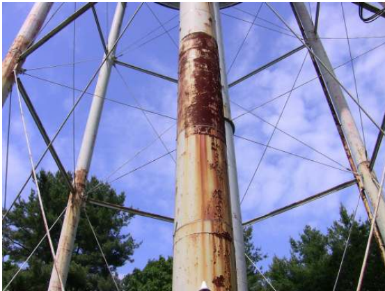
Extensive coating failure along the outer face of one of the leg columns.
