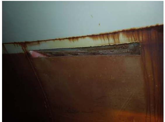
The rough cut opening of the overflow weir box just below the roof to knuckle junction.
