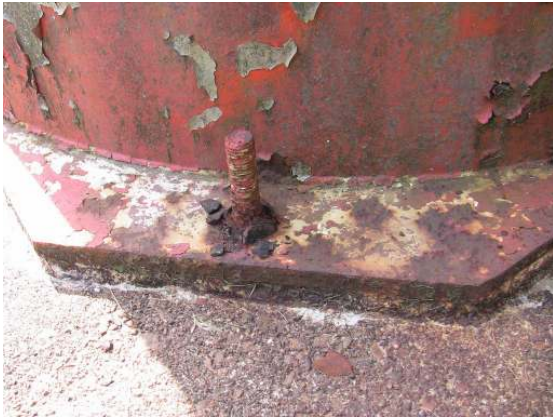
Metal fatigue has resulted in almost complete loss of an anchor bolt retention nut at the base of a support column.
