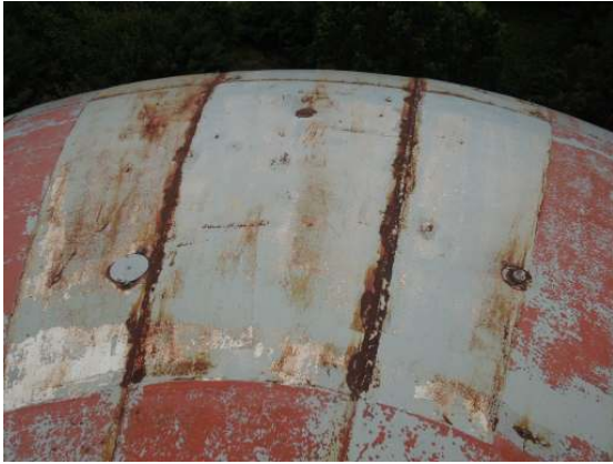
Failure of the roof coating has resulted in medium to heavy surface corrosion along the roof plates and weld seams.
