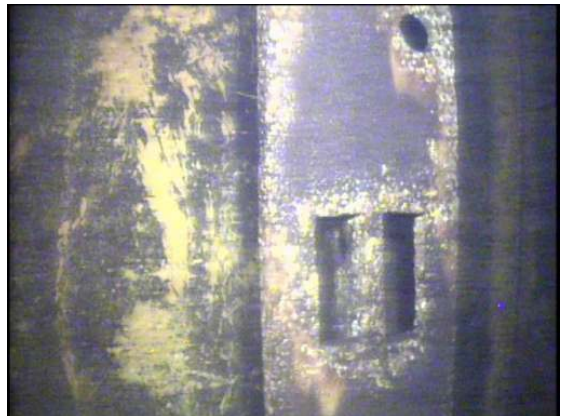
Heavy blistering and scattered corrosion along the vertical shell stiffeners.
