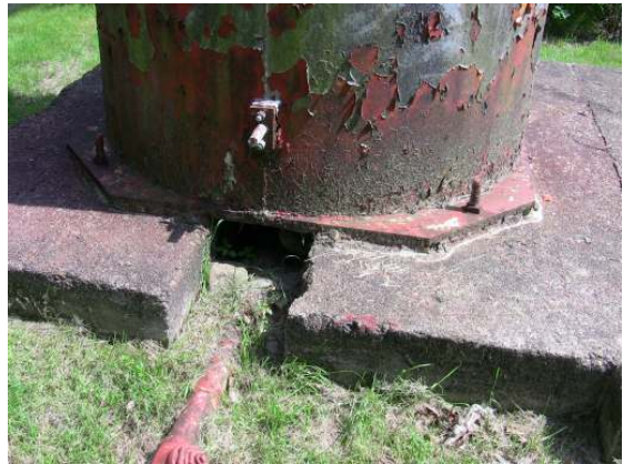
Showing the valve stem and piping at the base of the riser. The riser base plate and anchor bolts are exhibiting heavy corrosion.
