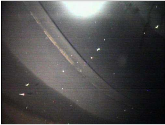
Additional areas of corrosion visible along the underside of the upper shell stiffener.
