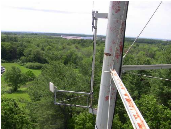
Antenna equipment mounted to bracket assemblies along the tank support structure.
