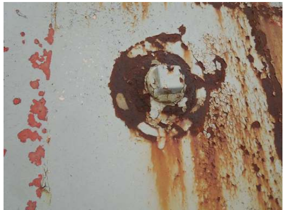
Showing a roof rigging coupling with installed plug, but coating failure and heavy corrosion along the adjacent plate surfaces.
