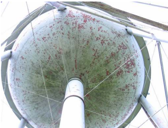
An overall view of the tank bowl surfaces indicating the widespread top coat failure and surface soiling.
