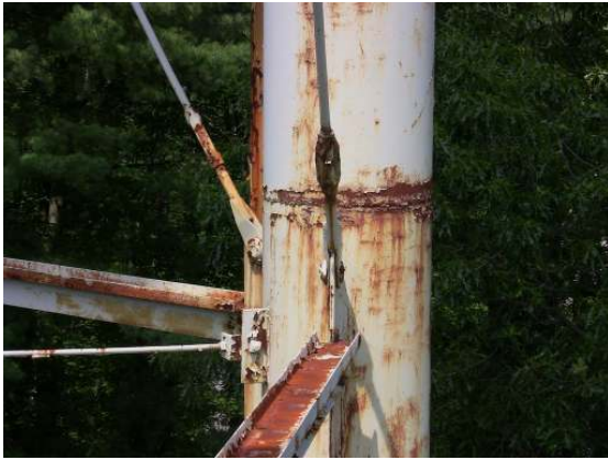
Extensive peeling and delamination at all interfaces as well as surface corrosion throughout the support columns, struts and rods.
