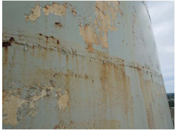
Showing widespread cracking and delamination of the shell coatings with associated rust formation.
