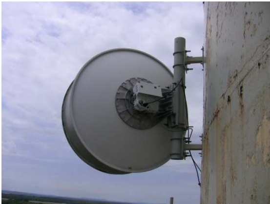
There are a number of antennas secured to stud welded mounts on the shell surfaces of the tank.
