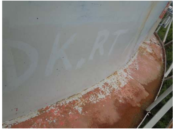
Graffiti evidence that unauthorized personnel have gained access to the upper tank surfaces.
