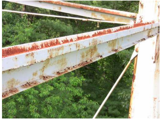
Widespread coating failure and surface corrosion along a horizontal strut of the support structure.
