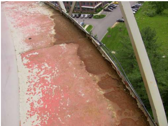
The top deck of the balcony is in poor condition, with widespread coating failure and surface corrosion.
