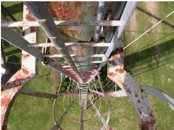
The leg column ladder is exhibiting widespread coating failure as observed on the surrounding column surfaces.
