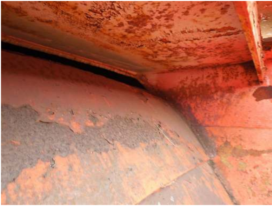
Showing coating failure along the interior of the weir box and the opening into the water chamber.
