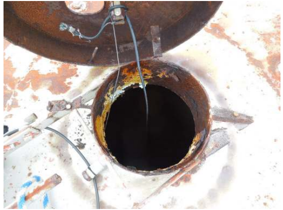
The interior of the finial stub is exhibiting extensive corrosion but should support installation of a new vent assembly.
