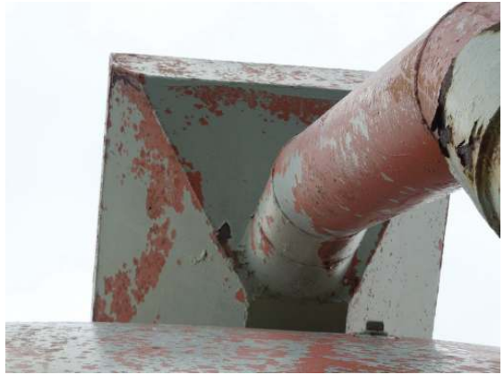
Showing widespread top coat failure and some surface corrosion along the exterior of the weir box and upper overflow pipe.
