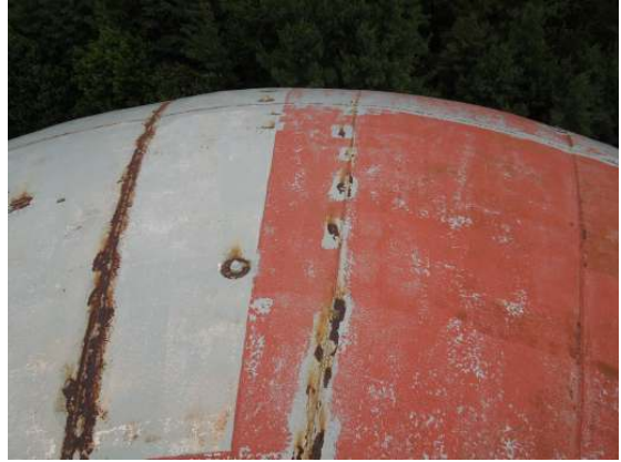
Extensive coating failure to multiple interfaces was noted throughout the roof surfaces.
