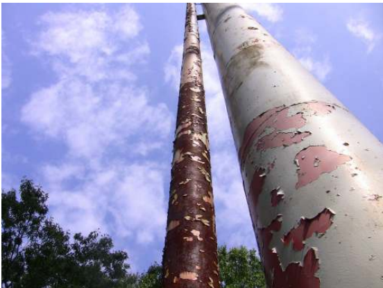
Almost complete coating failure and uniform surface corrosion along the overflow pipe along the leg column.
