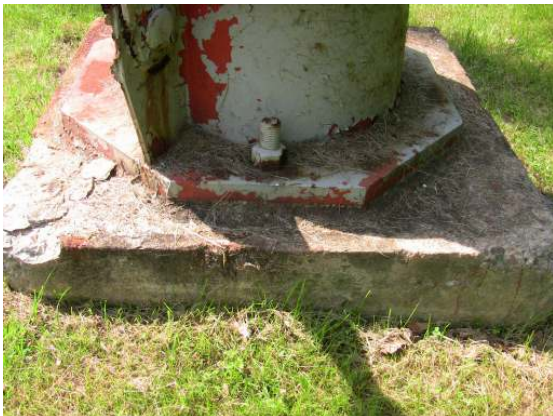
Coating failure and corrosion of the leg column anchor bolts. The concrete footings are generally sound, with only minor surface spalling.
