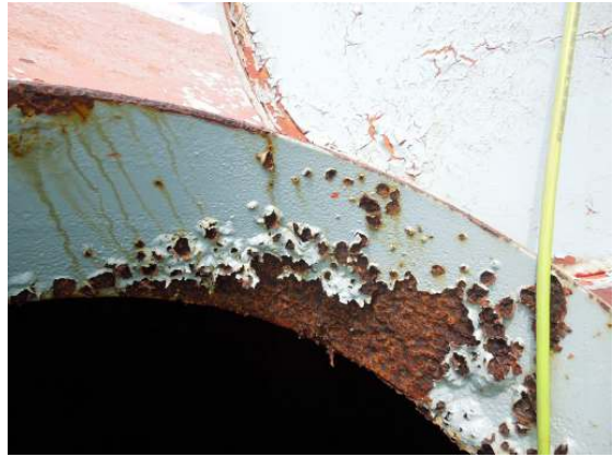
Showing coating failure and heavy corrosion of the interior hatch neck with measureable metal loss noted.
