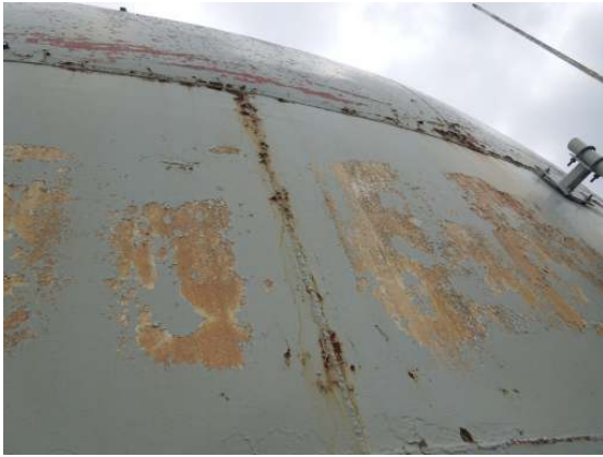
Coating failure is evident along multiple different interfaces along the shell surfaces.
