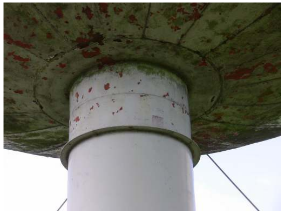
Continuation of some top coat failure along the upper surfaces of the riser.
