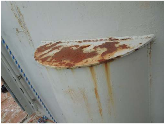
Coating failure and surface corrosion along the top face of a leg column insert.
