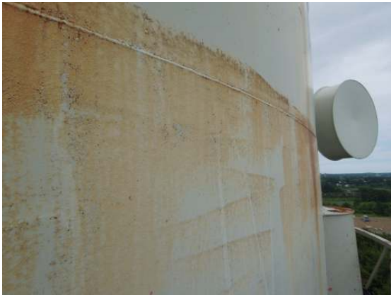
Additional areas of coating breakdown and light rust bloom along the exterior shell surfaces.
