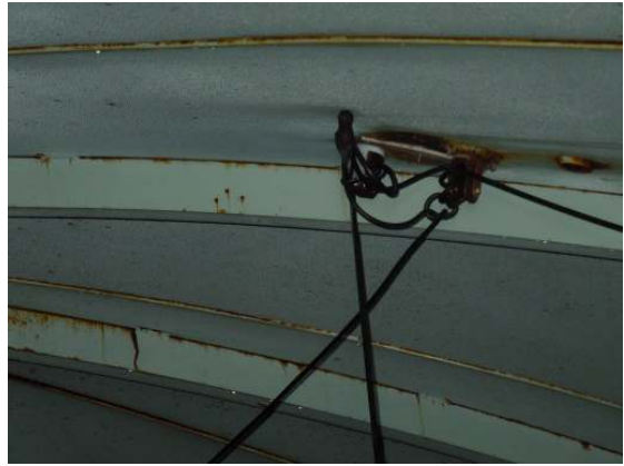
Corrosion along lap seams, junctions with the roof rafters and along the cathodic and rigging penetrations.
