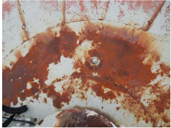
Extensive coating failure and surface rusting along the center roof plate surfaces.
