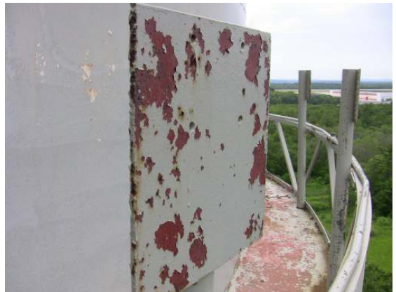
Widespread top coat failure extends to the leg column inserts at balcony level.
