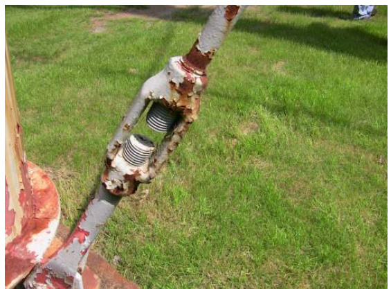
Extensive coating failure and surface corrosion along a lower level sway rod turnbuckle.
