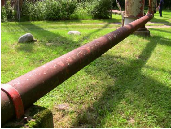
The horizontal segment of the overflow pipe is exhibiting complete coating failure and uniform surface corrosion.
