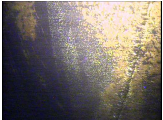
Additional area of heavy blistering and surface corrosion along the shell.
