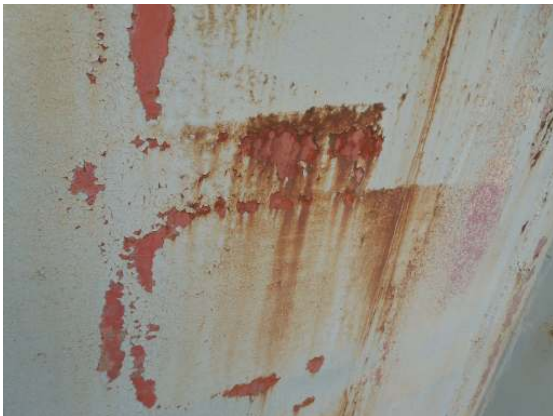
An area of heavy cracking of the top coats and light rust staining or bleedthrough along the surrounding coatings.
