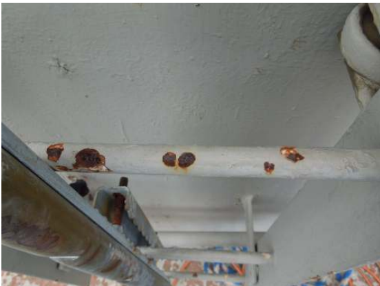
Showing scattered areas of coating failure and corrosion along the shell ladder rungs.
