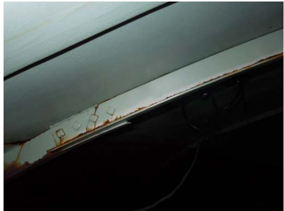
Additional areas of corrosion along the top face of the rafter lower leg and outer roof bolted connections.
