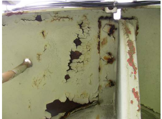
Showing a localized area of coating failure and corrosion along the underside of the balcony deck and a support bracket.
