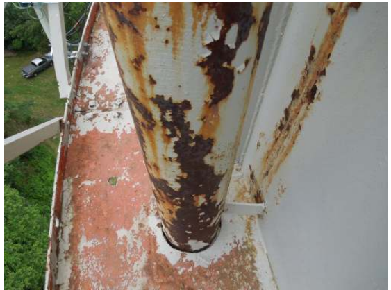
Widespread coating failure and surface corrosion where the overflow pipe extends through the balcony deck.
