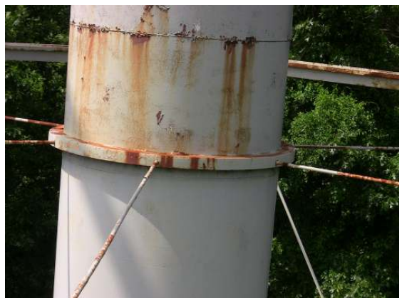
Coating failure and surface corrosion along the riser stiffener ring for the radial support rods.
