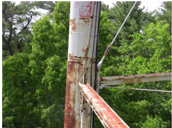
Widespread coating failure and surface corrosion along the tank support structure.
