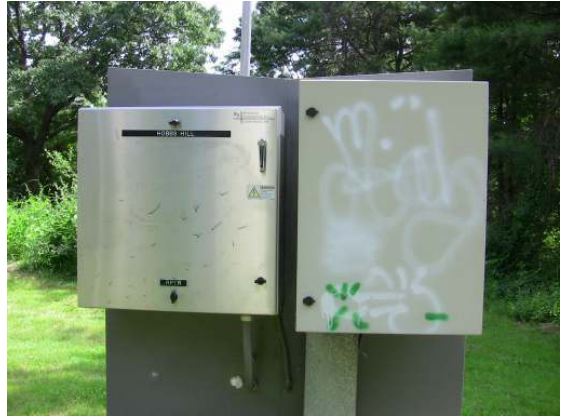
Tank controls on a free standing platform on the tank site.
