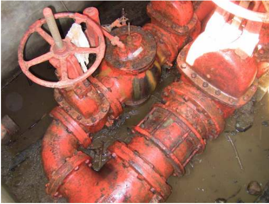
The coatings on the interior piping are in poor condition, and there is some standing water.
