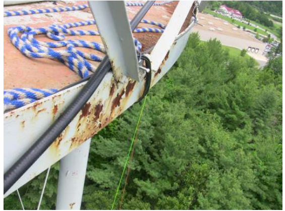
Additional areas of cracked and delaminated coatings along the outer face of the balcony kick plate.
