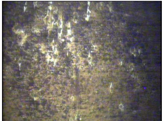
An area where the rupture of a number of small blisters has resulted in corrosion of the underlying steel.
