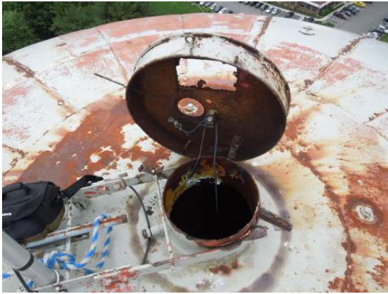
Extensive metal loss along the cap support brackets allows the cap to be removed easily with no screen present.
