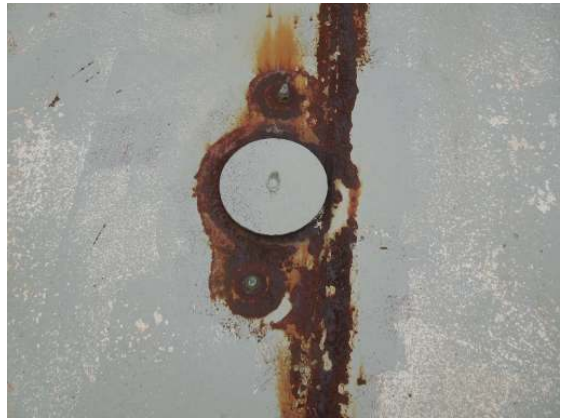
A series of cathodic port covers and insulator bolts are present throughout the roof that are intact but heavily rusted.
