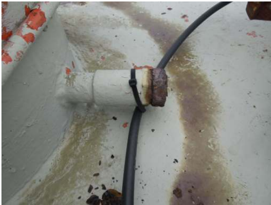
A small penetration in the side of the finial stub is secured with a plug that is uncoated and severely rusted.
