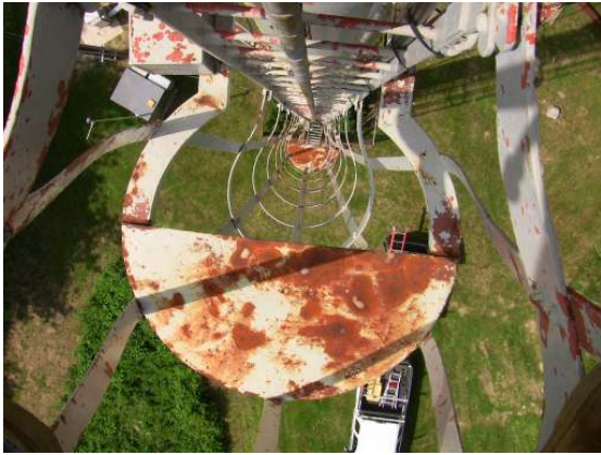
Coating failure and surface corrosion along the top face of one of the leg column ladder rest platforms.
