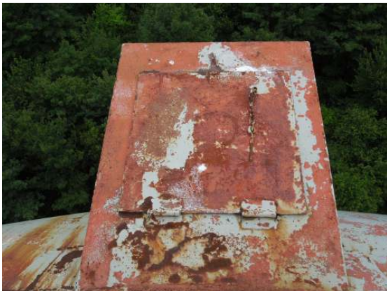
The top hatch of the overflow weir box is in poor condition, with complete failure of the cover hinges.
