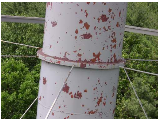
Widespread top coat delamination but only minor corrosion along the riser surfaces.
