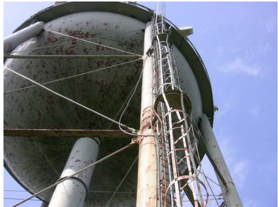
The leg column access ladder is equipped with a cage, rest platforms and a notched rail safety climb system.
