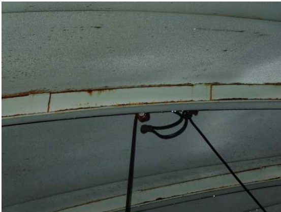
Significant coating failure and corrosion was noted along the top faces of the angle lower leg of the rafter.
