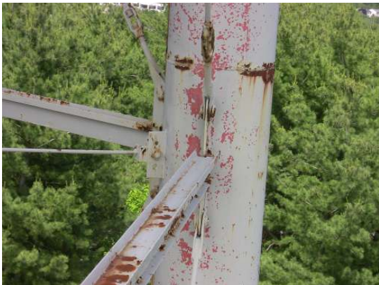
Coating delamination at multiple interfaces as well as localized medium to heavy corrosion along the support columns.
