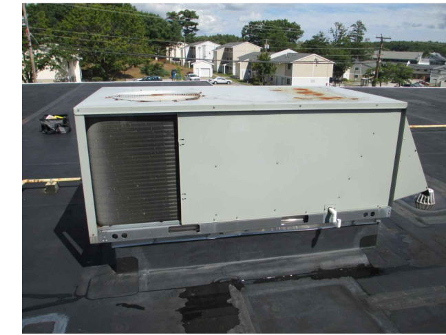
⑫ RTU 2 (East View)
