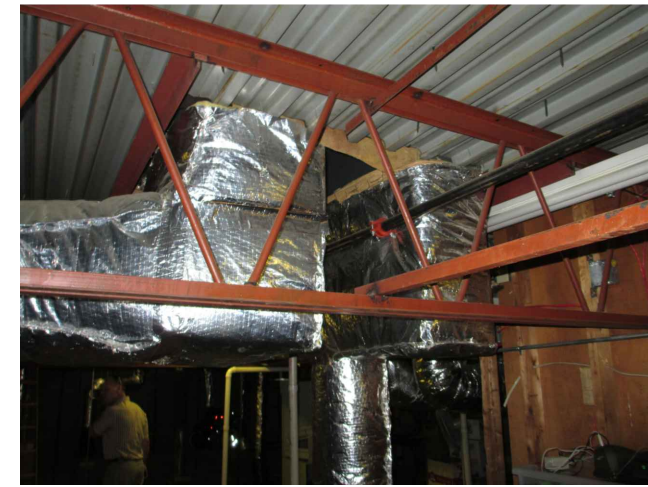
⑧ RTU Ducting
