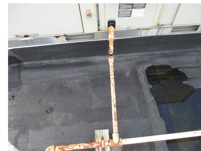
⑱ RTU 3 Gas Supply Connection
