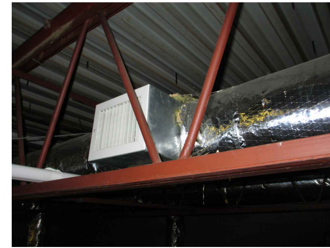
⑨ RTU Ducting
