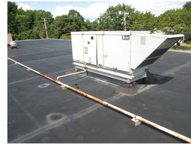
⑩ RTU 3 (Northeast View)
