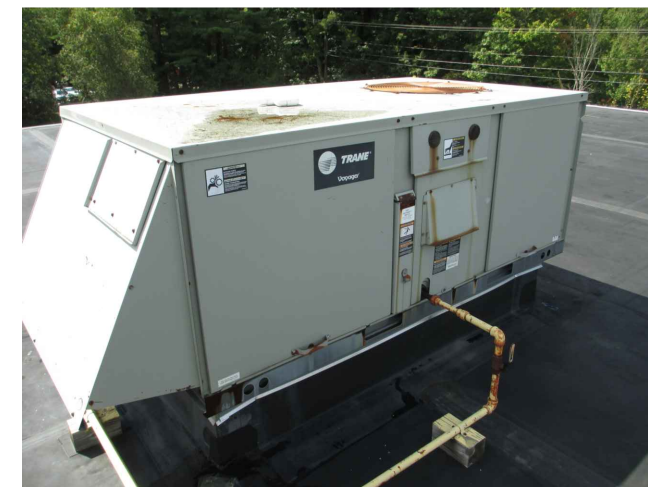
⑬ RTU 1 (Northwest View)
