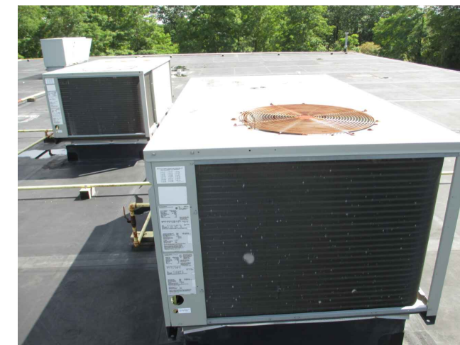
⑭ RTU 1 & RTU 2 (South View)
