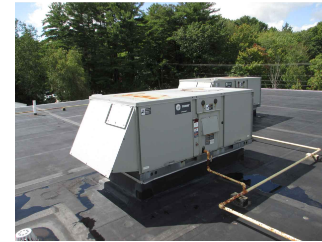
⑪ RTU 2 (Northwest View)
