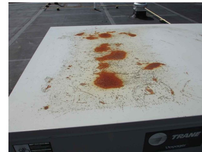
⑮ RTU 3 Corrosion
