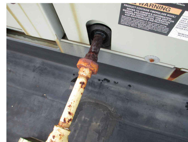
⑲ RTU 1 Gas Supply Piping Connection
