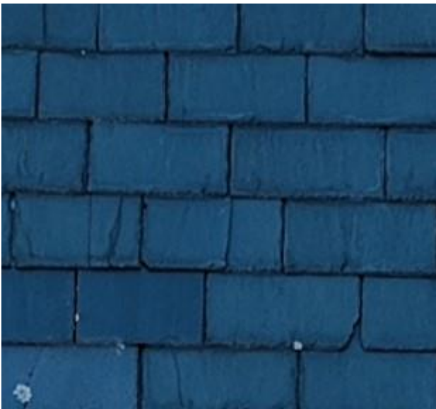
Example of a typical BLUE dot condition. Cracked slate typically along the drip line and potentially causing a waterproofing issue.
