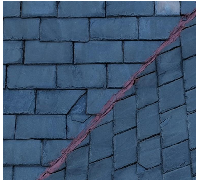
Example of a typical YELLOW dot condition. Damaged and/or in need or repair.
