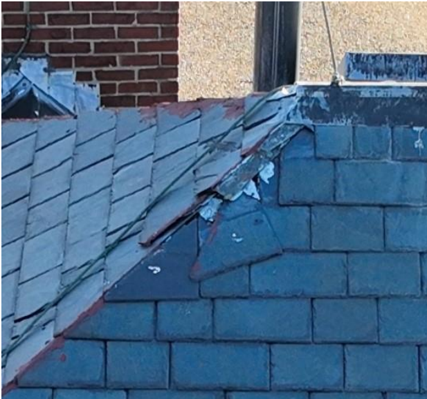
Example of a typical RED dot condition. Missing or in danged of falling off the building.
