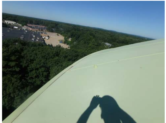
Showing junction between roof plates and rim angle to be sealed and in sound structural condition
