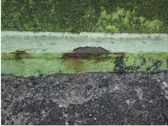
Shows medium to heavy grade surface rust along the floor plate extension
