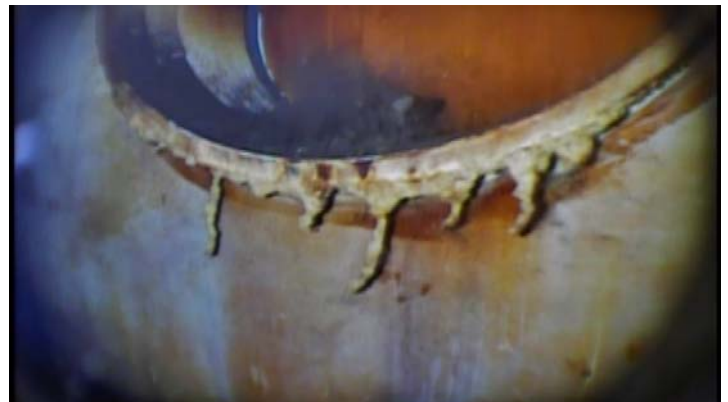
Showing evidence of heavy corrosion along the bottom edge of the manhole neck
