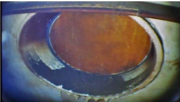
Showing the interior face of the 1st of (3) shell manholes to be intact and structurally sound
