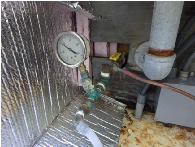
Showing the presence of a pressure gauge and a sample tap located within the telemetry box
