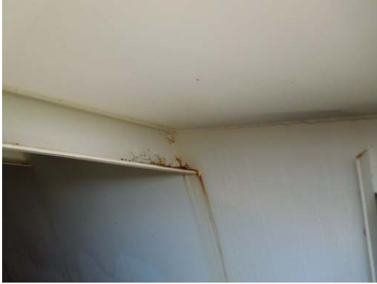
Coating degradation on the ends of the rafters has resulted in medium to heavy rust formation adjacent to the shell plate
