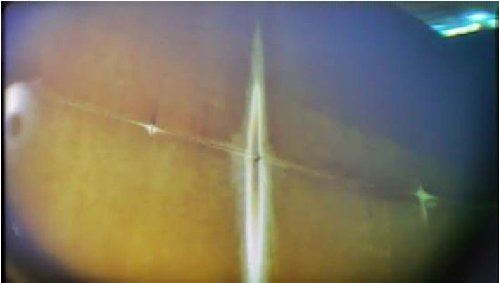
Showing isolated areas of small to medium rust tubercle formation along the upper shell rings
