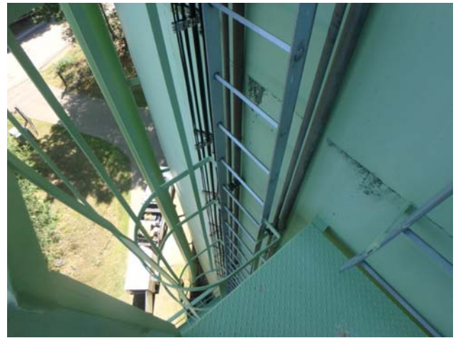
Showing lower sections of stainless steel access ladders to be intact and structurally sound
