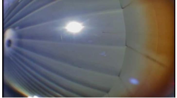
Coating along the upper shell surfaces appears to be in good condition with only heavy staining evident
