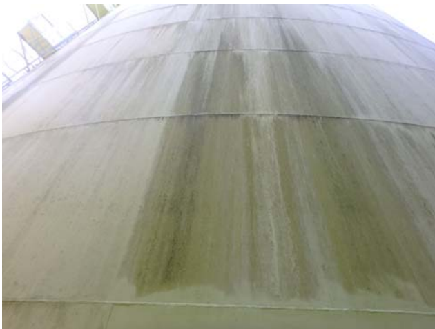
Coatings along the shell surfaces are in generally very good condition however heavily soiled
