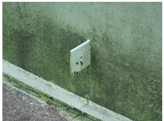
There is a series of unused ground lugs welded to the bottom shell ring which are showing medium to heavy rust formation where the coating is damaged
