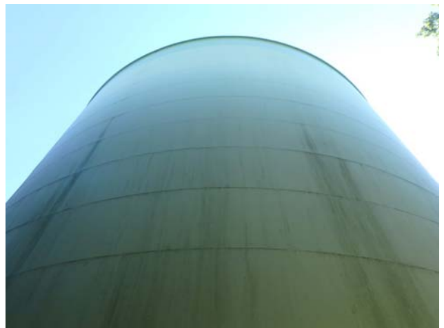
Coatings along the shell surfaces are in generally very good condition with minimal degradation evident
