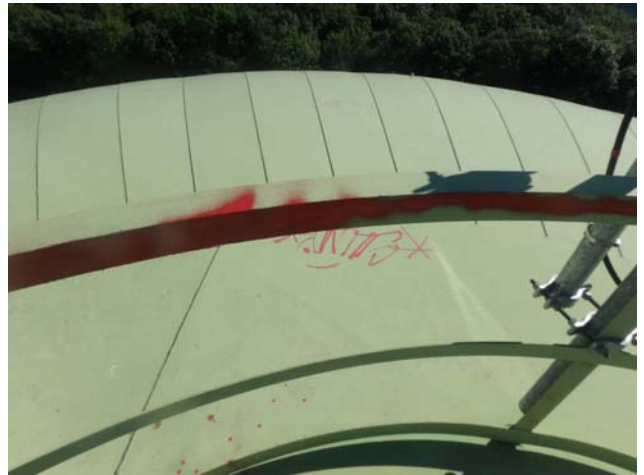
Showing handrail assembly surrounding the center of the roof to be intact and structurally sound
