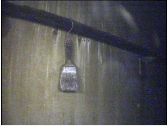
A paint brush has been left inside the tank after past maintenance operations
