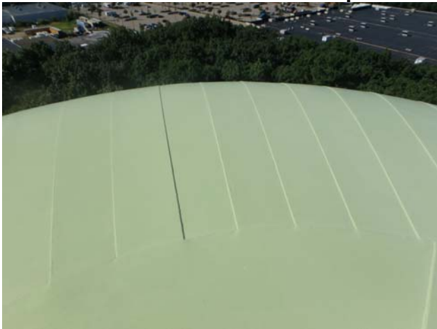
Showing coatings along the roof exterior surfaces to be in generally good condition
