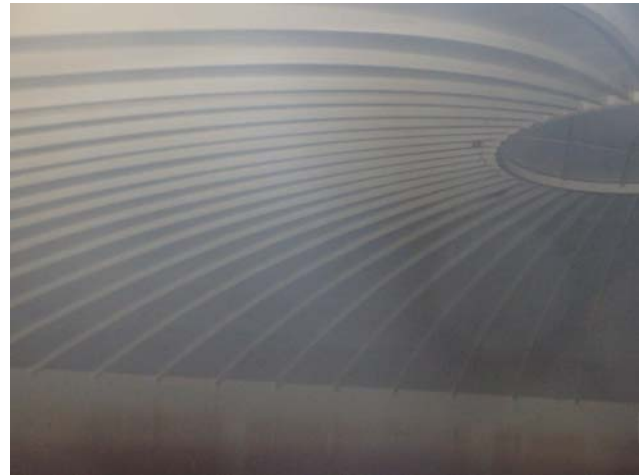
Showing the coatings along the underside of the roof to be in very good condition with only minimal degradation evident
