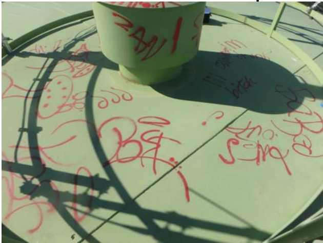
Showing additional graffiti applied to the exterior of the roof since our last inspection
