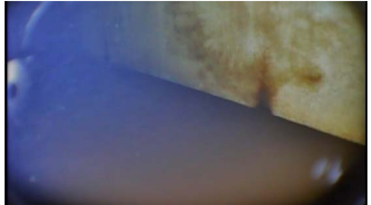
Showing scattered areas of heavy rusting along the shell to floor junction
