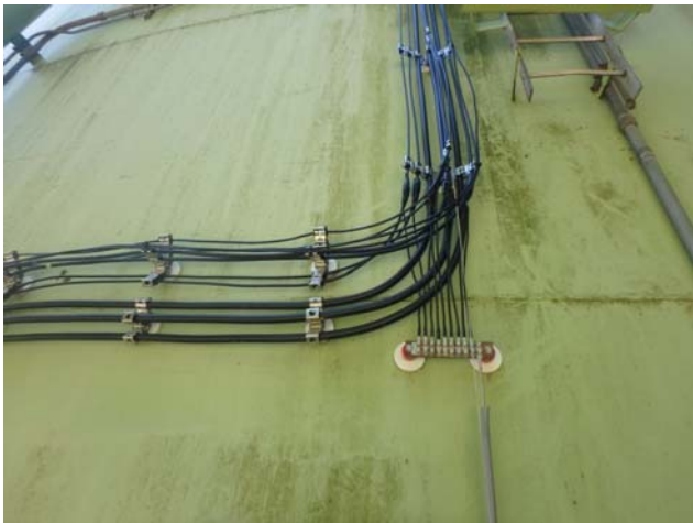
Showing run of antenna cables and grounding wires attached to the shell of the tank by magnetic mounts
