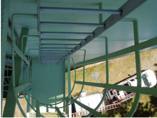
The shell ladders are uncoated stainless steel but the cage and platforms are painted mild which are in good condition
