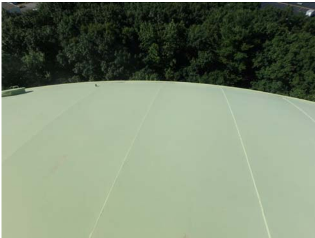
Showing coatings along the roof exterior surfaces to be in generally good condition
