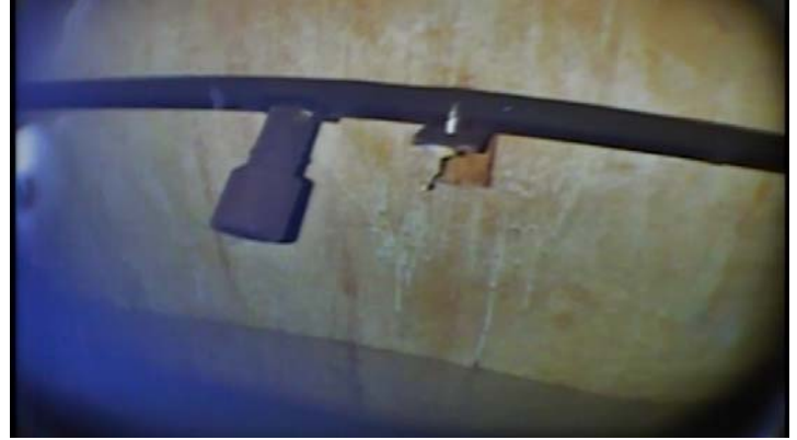
Showing the bubbler system to be intact however not active
