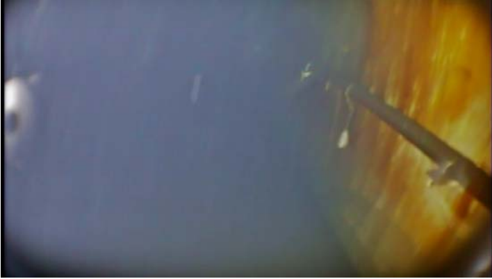
Showing evidence of heavy corrosion taking place along bubbler support brackets
