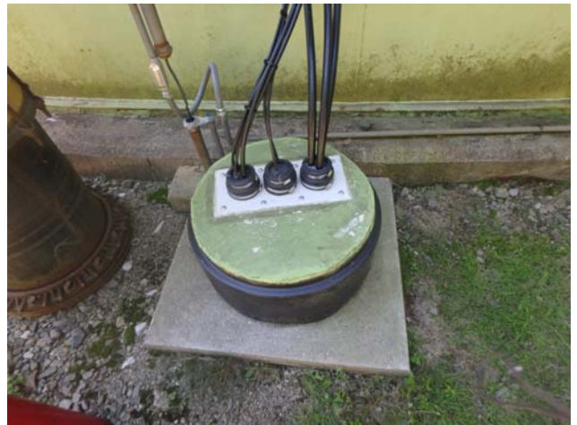
Showing antenna cables extending down into a capped underground conduit
