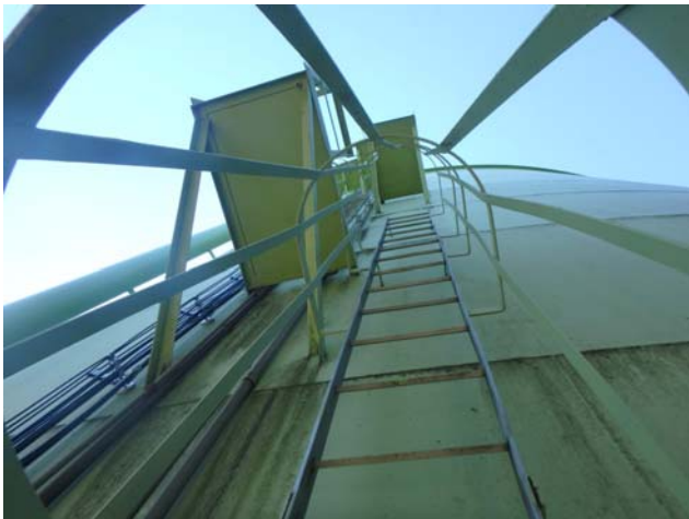
Showing bottom section of shell access ladder assembly to be intact , structurally sound and in good condition
