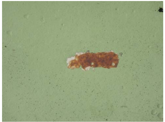
Showing small area of coating delamination along roof resulting in the exposure of the steel substrate and minor rusting
