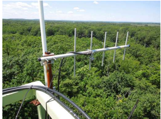
SCADA and whip antennas and associated coax cables are attached to the upper platform handrails
