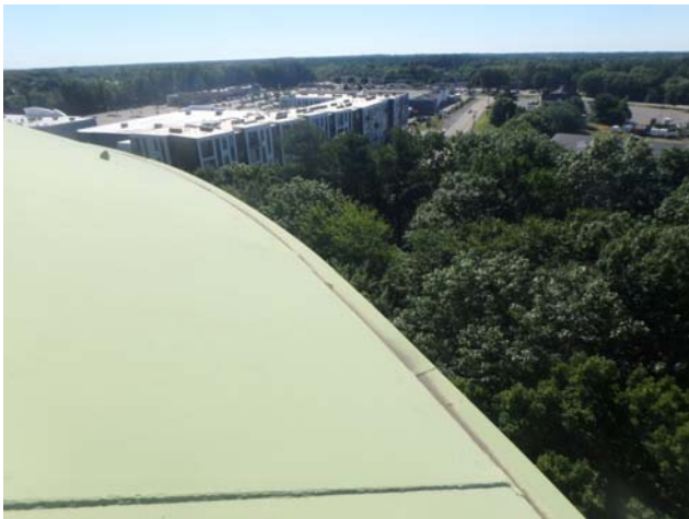
Showing junction between roof plates and rim angle to be sealed and in sound structural condition
