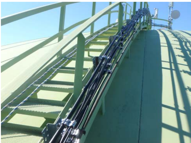
Showing antenna coax cables attached to the side of the roof stairway assembly
