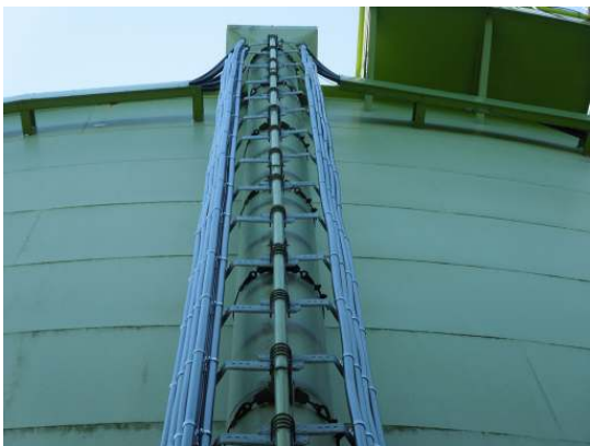
The majority of the overflow pipe is covered with coax cables and mounting brackets
