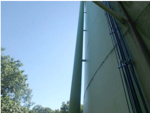
Showing overflow assembly to be intact, structurally sound and in good condition
