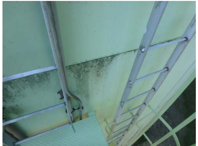
Showing additional section of shell access ladder to be intact and structurally sound
