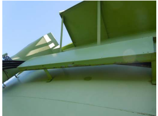
The coatings on the horizontal portion of the enclosed cable trays is delaminating exposing the underlying bright metal surface
