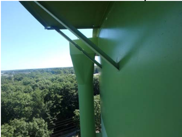
Showing overflow assembly to be intact, structurally sound and in good condition
