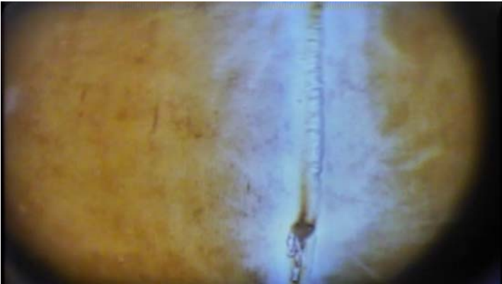
Showing isolated area of small rust tubercle formation along interior vertical weld seam
