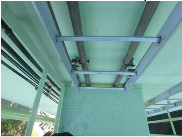
Showing conduit impeding clearance in behind shell access ladder
