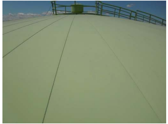
The majority of the roof coating is in sound condition with little degradation observed
