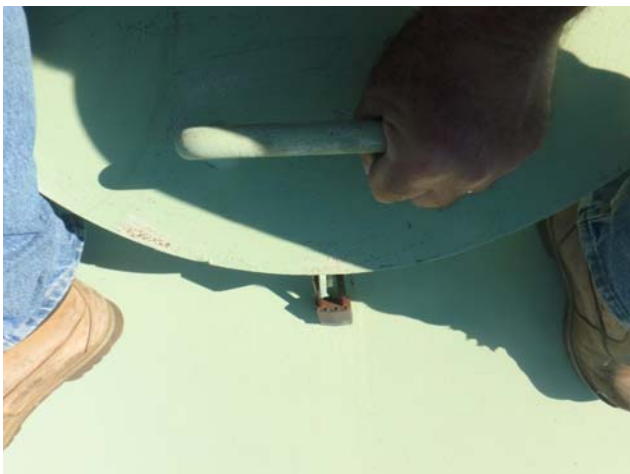
Showing secondary roof hatch cover closed and locked prior to and after this inspection
