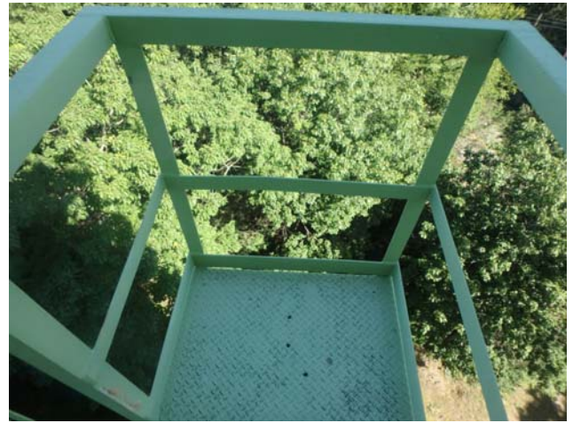
Showing shell access ladder platform to be intact, structurally sound and in generally good condition
