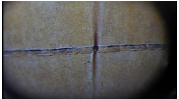
Showing isolated area of rust formation along interior horizontal weld seam
