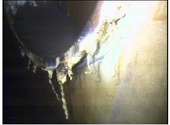
Shows corrosion along the neck portion of one of the shell manhole assemblies
