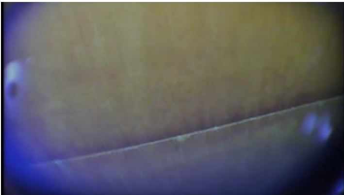
Coating along the upper shell surfaces appears to be in good condition with only heavy staining evident
