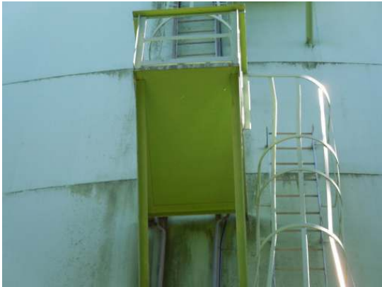
The coatings on the underside of the ladder platforms are in sound condition with little degradation observed
