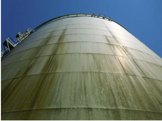
The majority of all shell surfaces are soiled and covered with algae growth
