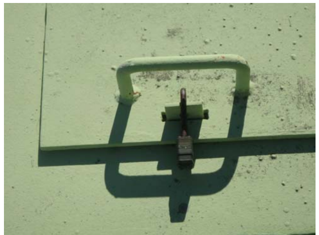
Showing weir box hatch cover closed and locked pre and post inspection
