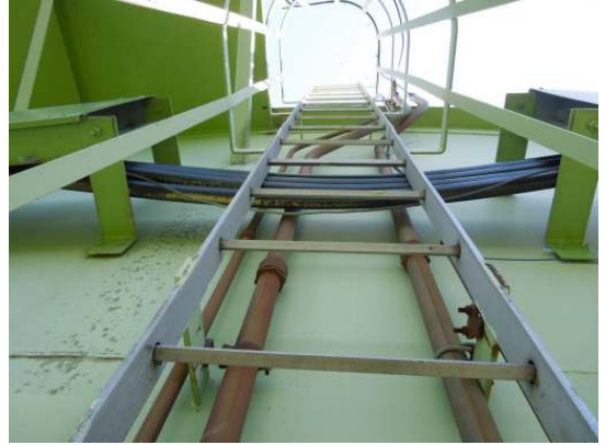
Shows miscellaneous conduits and coax cables behind the shell ladder at the top of the tank
