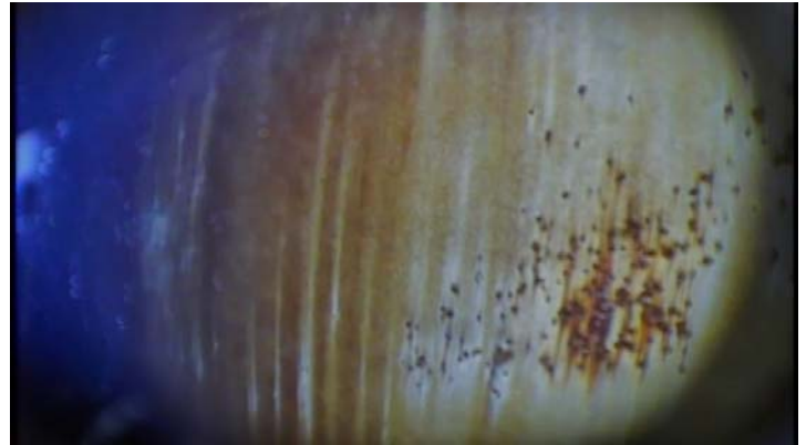
Showing evidence of blistering and scattered rusting along the interior surfaces of the bottom shell ring
