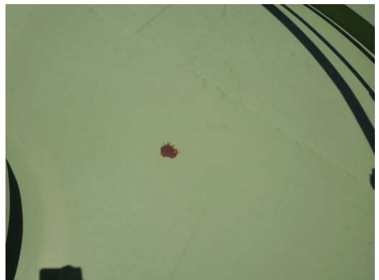
Shows a localized medium grade rust spot on center roof plate within the handrails
