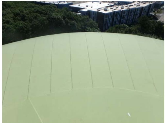
Showing coatings along the roof exterior surfaces to be in good condition with minimal degradation evident
