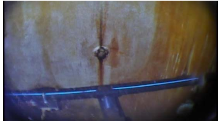
Showing heavy corrosion along the opening of a bottom ring penetration
