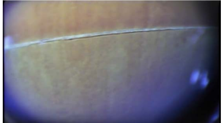
Coating along the upper shell surfaces appears to be in good condition with only heavy staining evident
