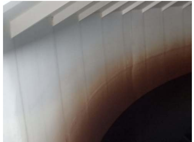
Coating along the shell surfaces above water level is in good condition with only staining evident
