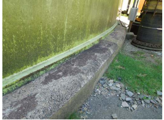
The majority of the grout between the foundation and floor plate extension is in sound condition
