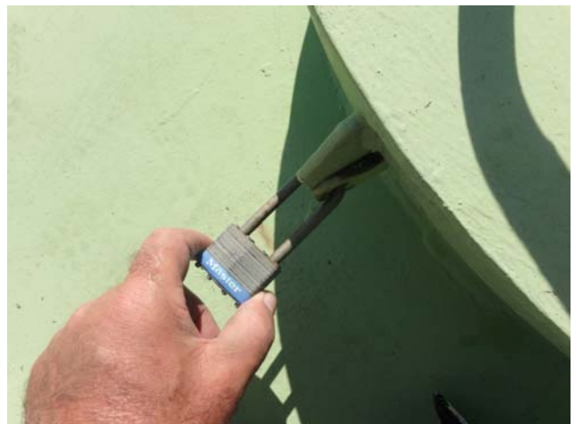
Showing cover of the primary roof hatch closed and locked post inspection
