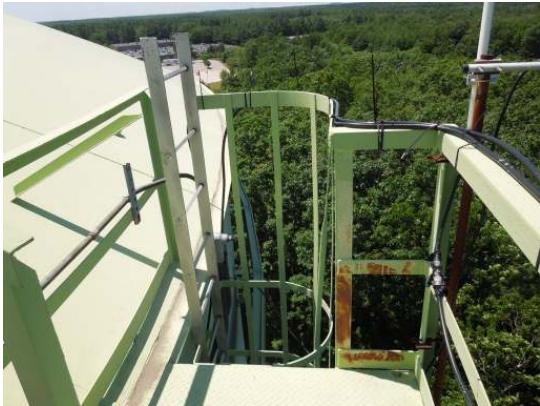
Shows localized area of corrosion on the handrail surfaces adjacent to the shell ladder
