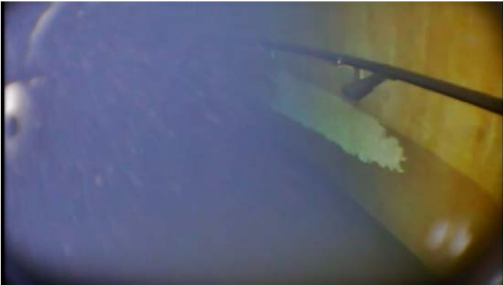
Showing additional section of the bubbler system to be intact and in visually good condition
