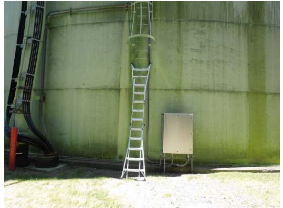
The shell ladder terminates approximately 10' above grade and is not equipped with a security gate
