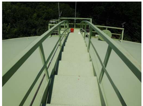
The majority of the coatings on the stair and handrail system are in good condition
