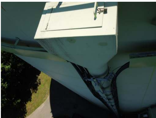
The exterior face of the weir box is soiled but does not exhibit any significant coating degradation
