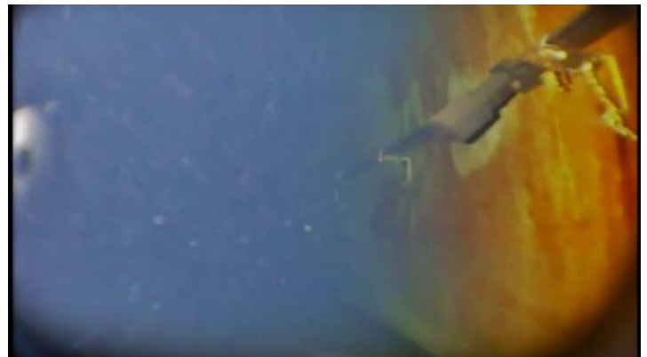
Showing evidence of heavy corrosion taking place along bubbler support brackets
