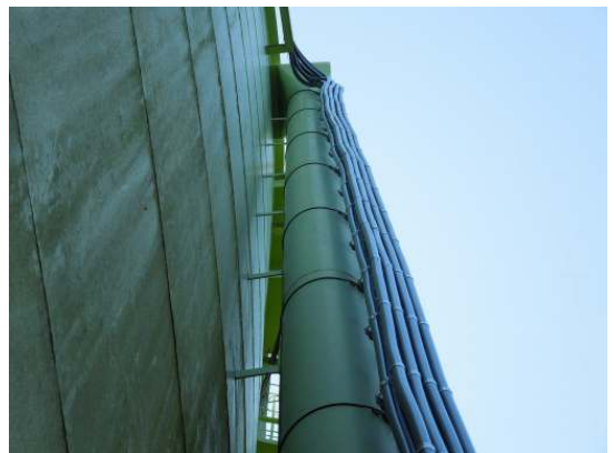
Coax cables are attached to the overflow pipe do not appear to have damaged the coating in any way
