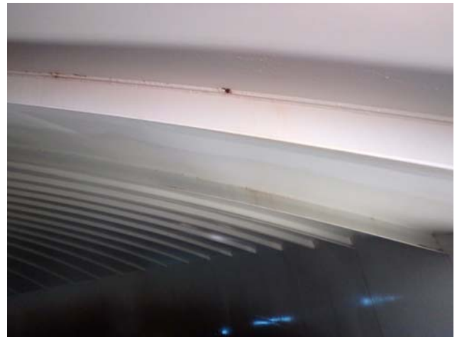
Showing evidence of minor coating degradation and rusting along underside of roof and junction with rafter
