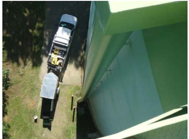
Showing antenna cables removed and overflow assembly recoated since our last inspection
