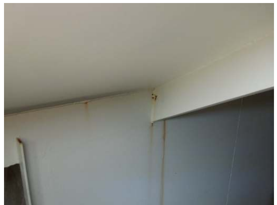
Shows scattered areas of corrosion on the ends of the rafters where welded to the shell
