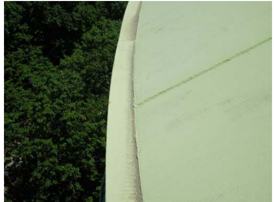
The outer edge of the roof is collecting dirt and there is minor light rust on the outer edge of the lip extension
