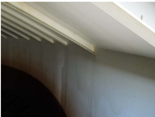
Corrosion along the ends of the rafters is staining the adjacent shell surfaces
