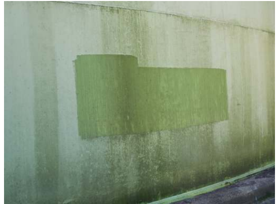
There is evidence of overcoat application on the bottom shell ring most likely to cover graffiti markings
