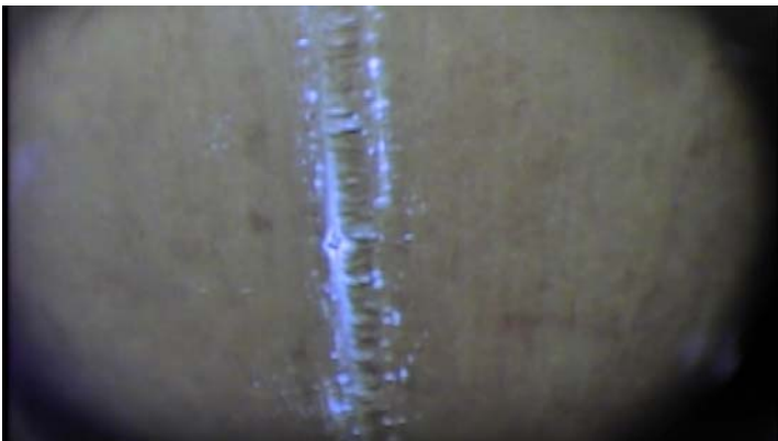
Showing evidence of minor degradation and rusting along vertical weld seam
