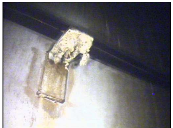
There is corrosion on the underside of the PVC support brackets
