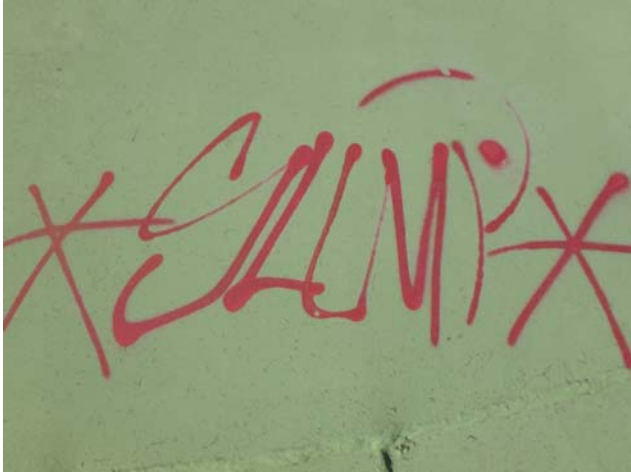
Showing new graffiti applied to the exterior of the roof since our last inspection
