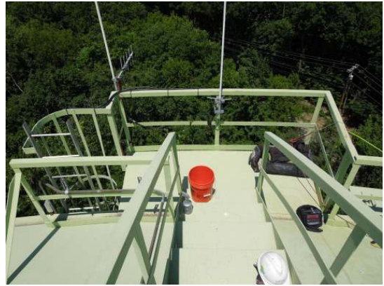
The majority of the coatings on the platform and handrails along the outer edge of the roof are in good condition
