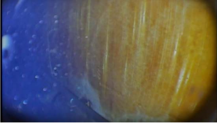
Showing additional coating degradation and rusting along the interior of the bottom shell ring
