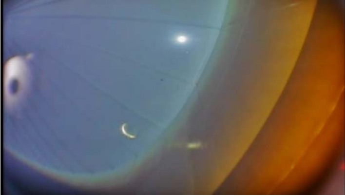
Coating along the upper shell surfaces appears to be in good condition with only heavy staining evident
