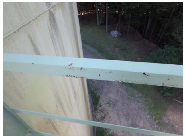
Showing minor coating degradation and rusting along one of the shell access ladder platforms
