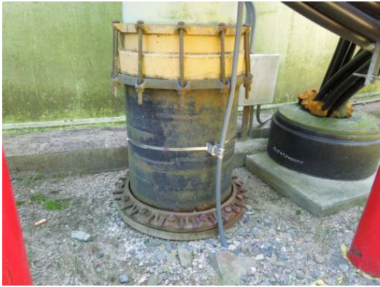
The overflow pipe is connected to underground piping which travels below grade before exiting at ground level
