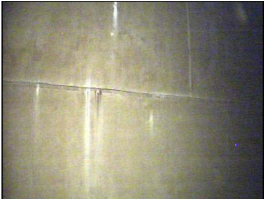
The majority of the coating below water level is in good condition
