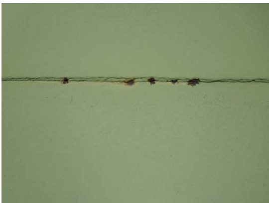
Localized areas of medium grade corrosion is present along several roof plate weld seams
