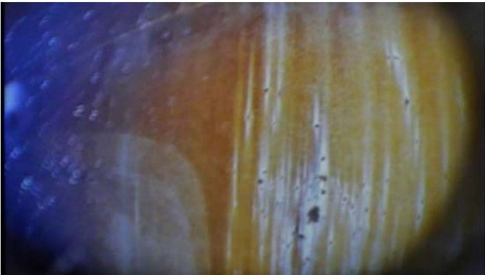
Showing evidence of blistering and scattered rusting along the interior surfaces of the bottom shell ring
