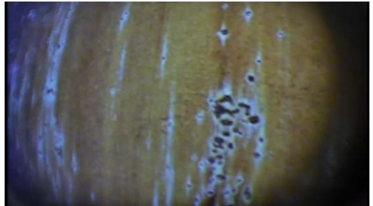
Showing evidence of blistering and scattered rusting along the interior surfaces of the bottom shell ring
