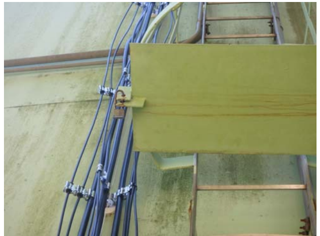
Showing security gate at bottom of access ladder cage to be closed and locked post inspection
