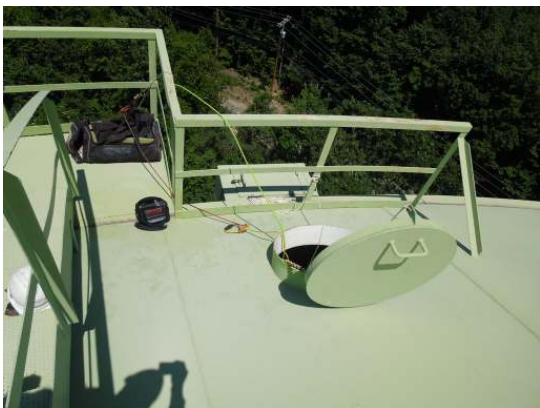
The primary roof hatch is enclosed with a handrail assembly for safety while accessing the tank interior
