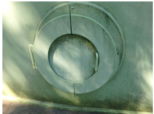
Showing the 1st of (3) shell manholes all of which appear intact and structurally sound
