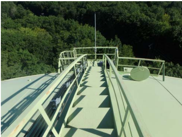
Showing coatings along the roof stairway assembly to be in good condition with only minor rusting evident
