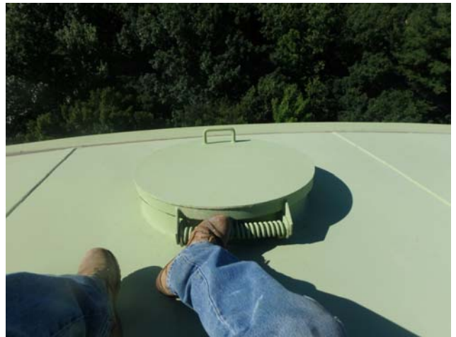
Showing secondary roof hatch assembly to be in good structural and sanitary condition
