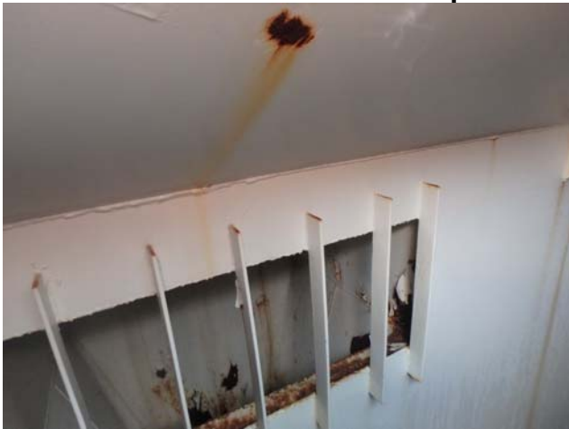
Showing evidence of extensive coating failure and rusting taking place along the interior of the weir box
