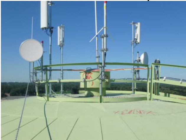
Showing assortment of antennas mounted to the roofs center handrail assembly
