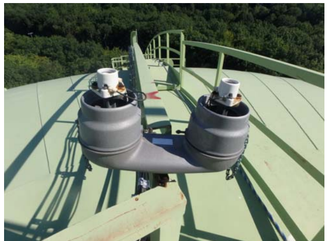
Showing FAA obstruction lighting missing bulbs and globes
