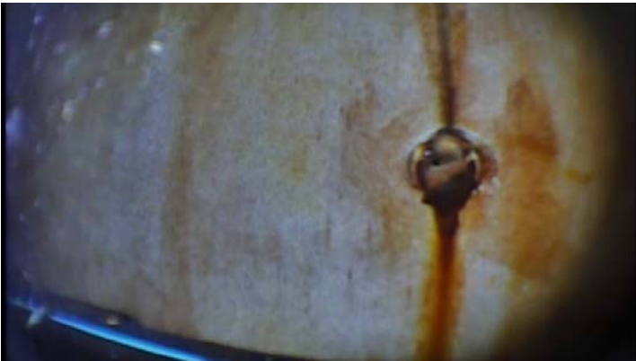
Showing heavy corrosion along the opening of a bottom ring penetration
