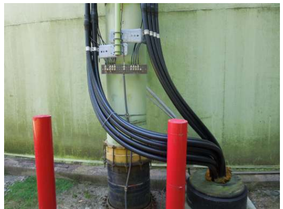
Shows bundles of coax cables prior to entering an underground conduit
