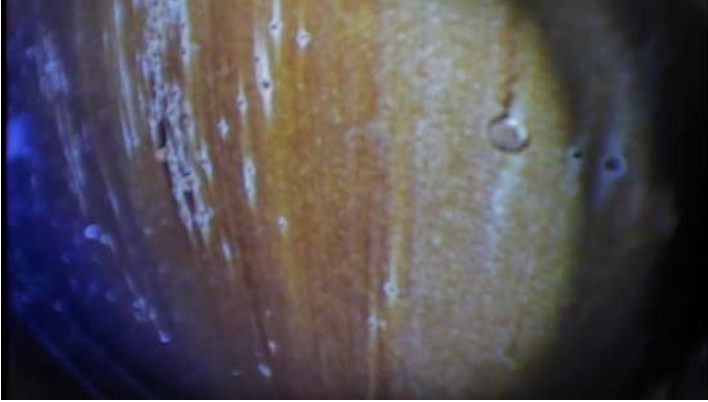
Showing evidence of blistering and scattered rusting along the interior surfaces of the bottom shell ring
