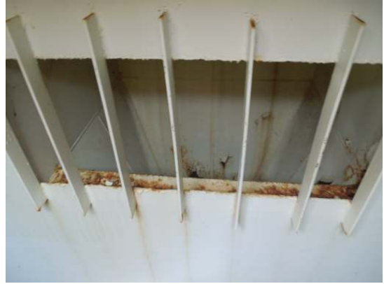
The coating on the interior faces of the weir box is in only fair to poor condition with extensive degradation noted
