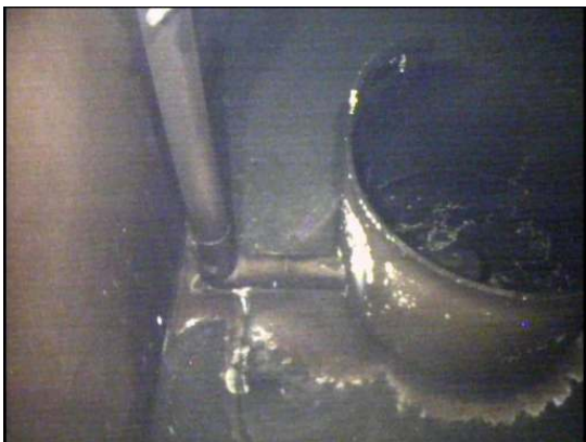
There is a PVC tube entering the side of the silt trap which then travels down the fill pipe
