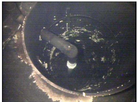
There is a PVC tube entering the side of the silt trap which then travels down the fill pipe
