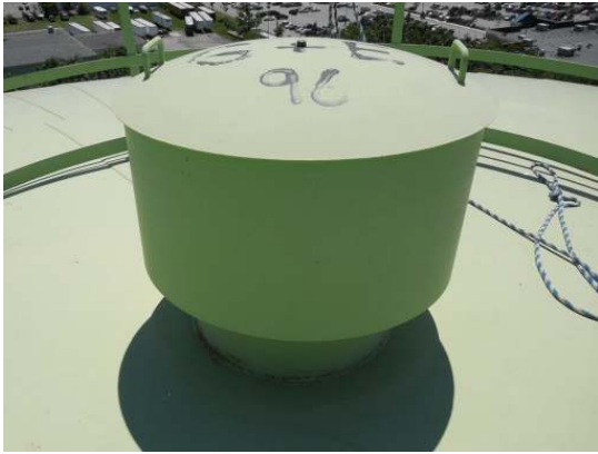
Shows the coatings on the finial vent cap are in good condition and there is evidence of old graffiti
