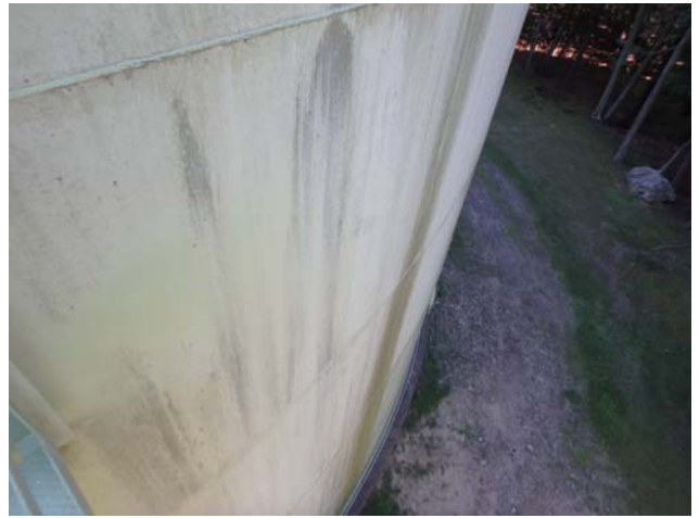
Coatings along the middle shell rings are in very good condition however heavily soiled
