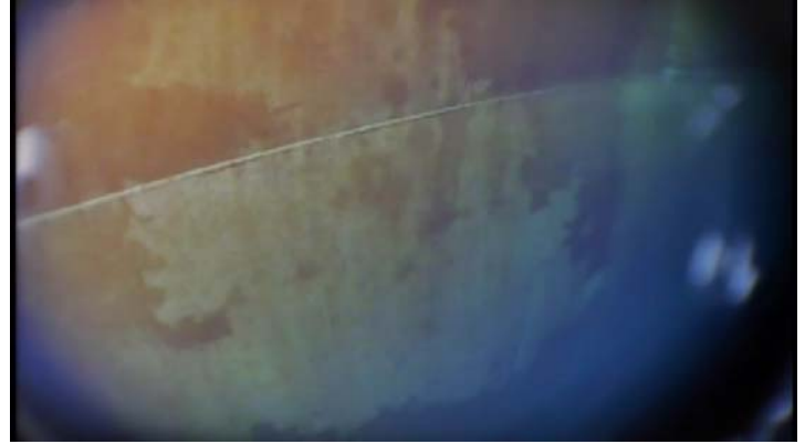
Showing coatings along the shell interior to be in generally good condition
