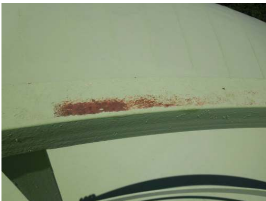
Shows areas of rust bleed through where the handrail coatings are heavily weathered
