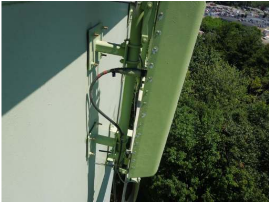
The antenna mounts are secured to the tank by stud welded bolts.
