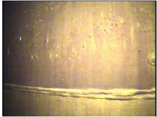
Shows an area of unbroken blistering on the shell surfaces
