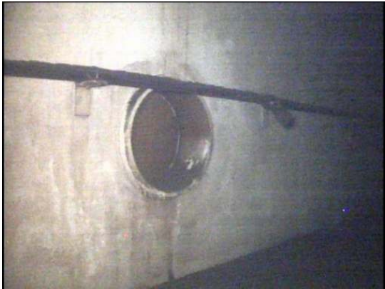
Shows what appears to be PVC piping attached to brackets adjacent to one of the shell manhole assemblies
