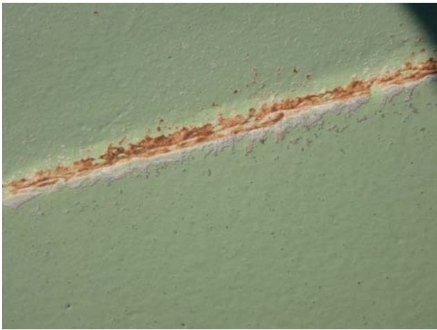
Showing minor coating degradation and rusting along exterior of the roof
