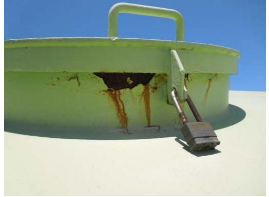
Shows areas of degraded coating on the secondary roof hatch neck exposing medium to heavy grade rust
