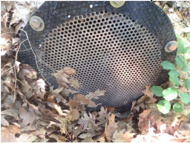
Showing discharge opening of overflow pipe fitted with a perforated metal screen
