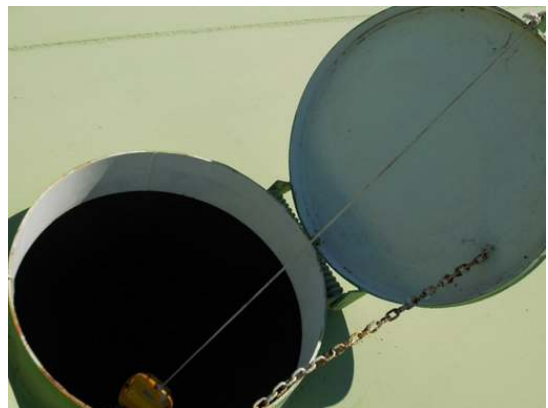
The coatings on the interior faces of the primary roof hatch are in generally good condition
