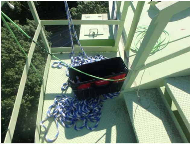
Showing top access platform to be intact, structurally sound and in generally good condition
