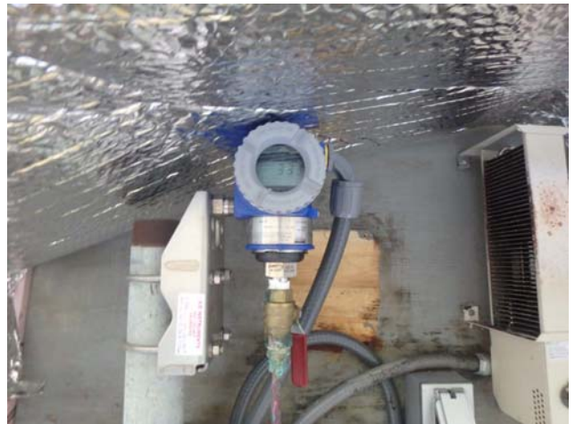
Showing a water level indicator located within the telemetry box
