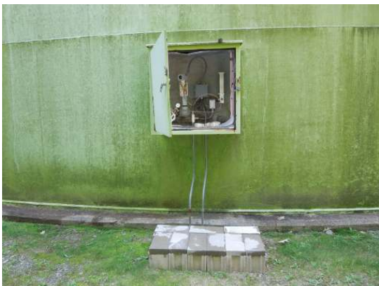
The telemetry box attached to the bottom shell ring appears to be in good condition
