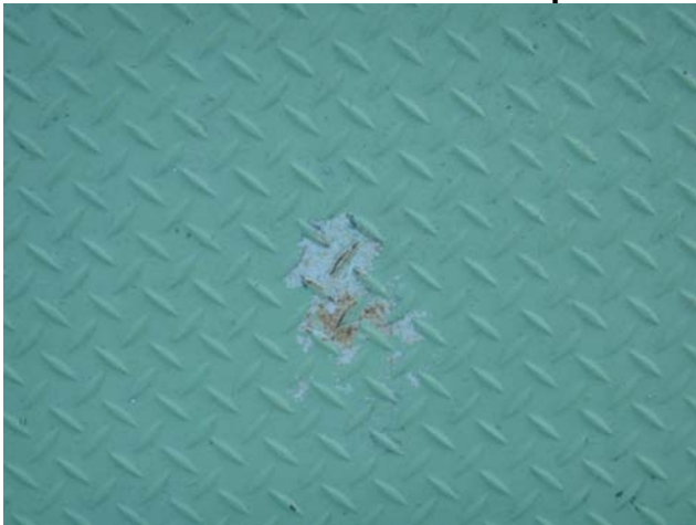
Showing minor coating delamination and rusting along one of the shell access ladder platforms
