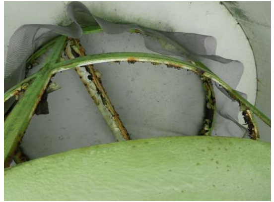
Shows medium to heavy grade rust on the vent framework and the screen is not covering the opening
