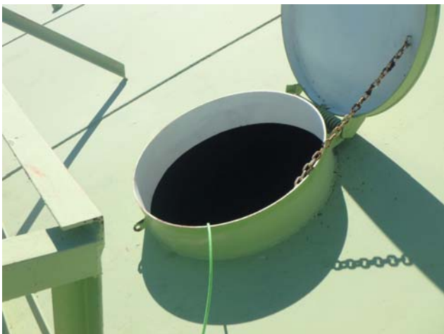
Showing coatings along primary roof hatch to be in good condition with minimal degradation and rusting evident
