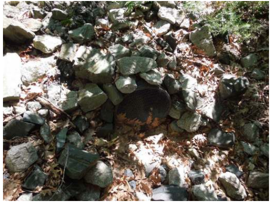
Shows an intact screen present on the underground portion of the overflow pipe where it exits the ground
