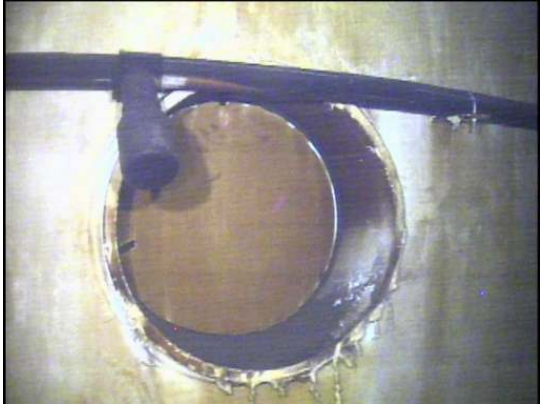
Shows one of two shell manhole assemblies exhibiting staining as well as areas of corrosion
