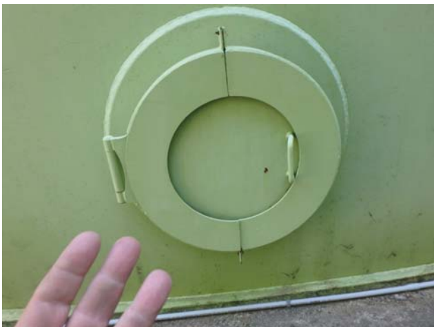
Showing the 3rd of (3) shell manholes all of which appear intact and structurally sound
