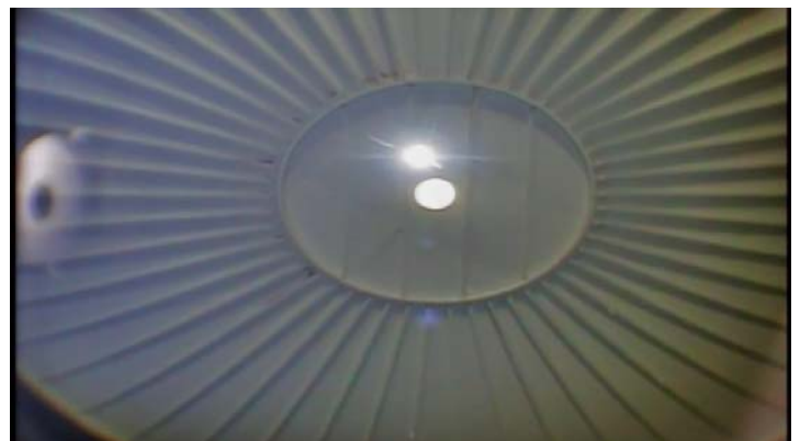
The coating along the underside of the roof appears to be in generally good condition with minimal degradation evident
