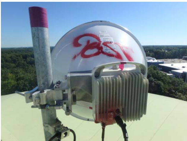
Showing one of many antennas attached to the roof center handrail assembly
