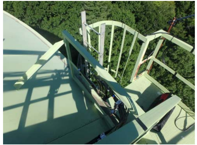
Showing top access platform to be intact, structurally sound and in generally good condition
