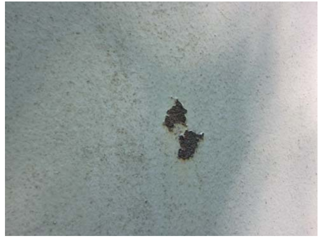
Showing isolated areas of coating failure resulting in exposure of the substrate and heavy rust
