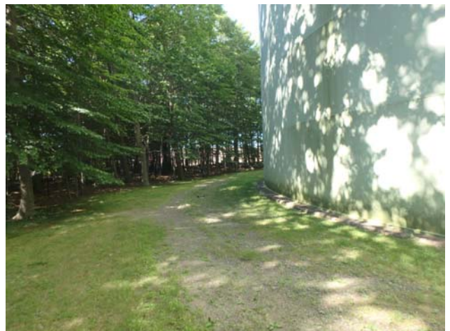
Showing coating along the lower shell rings to be in generally good condition
