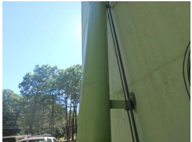
Showing overflow assembly to be intact, structurally sound and in good condition
