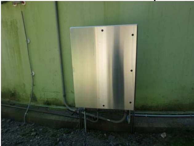
Showing what appears to be a sealed control cabinet for the obstruction lighting
