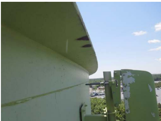
Shows a localized area of rust on the underside of the roof overhang
