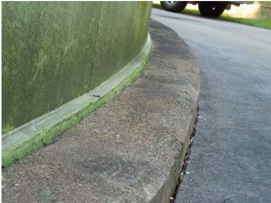
The top of the foundation is weathered to the point that the stone aggregate is exposed
