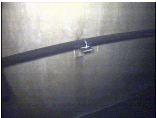
The PVC tubing is attached to brackets on the interior bottom shell ring with stainless steel u-bolts
