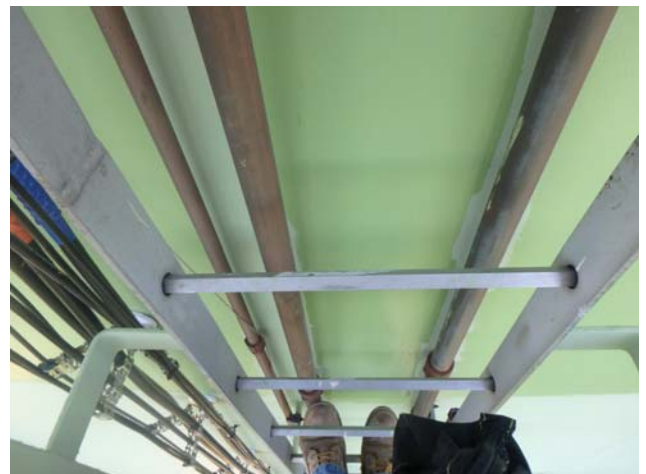
Showing shell stainless steel access ladder to be intact and structurally sound
