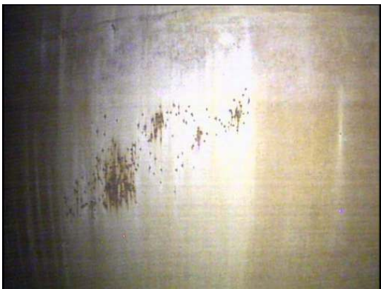
Shows a small cluster of broken blisters exposing light to medium rust on the exposed substrate
