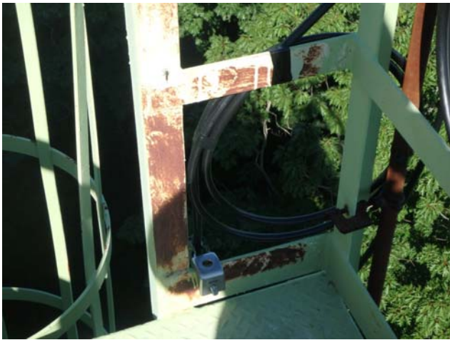
Showing localized area of coating degradation and rusting along platform handrail
