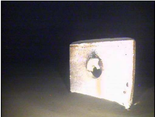
The rigging lug on the floor appears to be intact but there is evidence of heavy corrosion along the center hole
