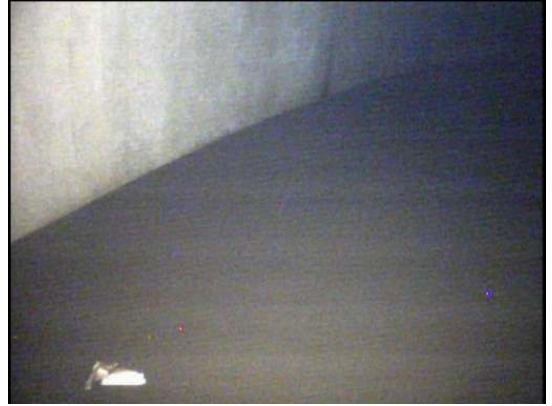
The floor is covered with a uniform layer of silt estimated to be approximately 1-2 inches deep
