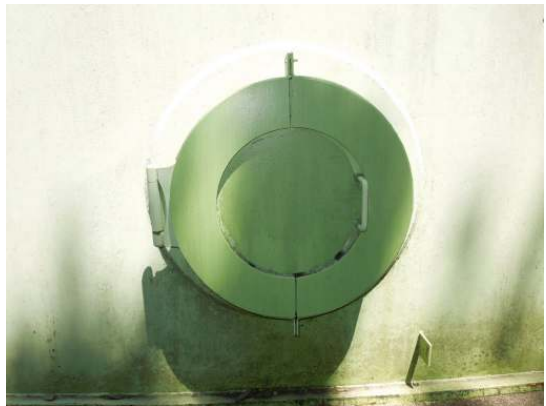
The coatings on the shell hatch assemblies appears to be in good condition with little degradation noted
