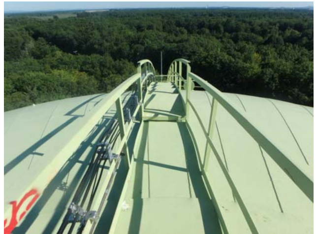
Showing coatings along the roof stairway assembly to be in generally good condition
