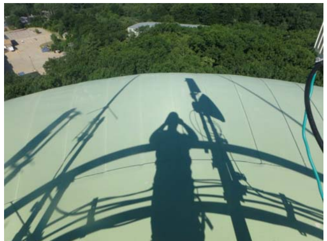
Showing coatings along the roof exterior surfaces to be in generally good condition
