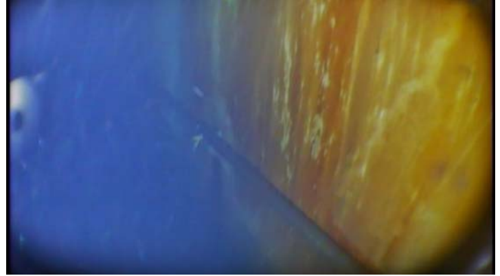
Showing additional coating degradation and rusting taking place along the interior of the bottom shell ring
