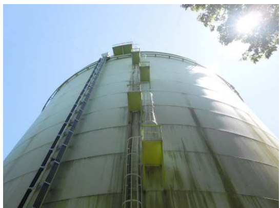
The tank is equipped with a series of offset ladders and platforms which appear to be in good condition
