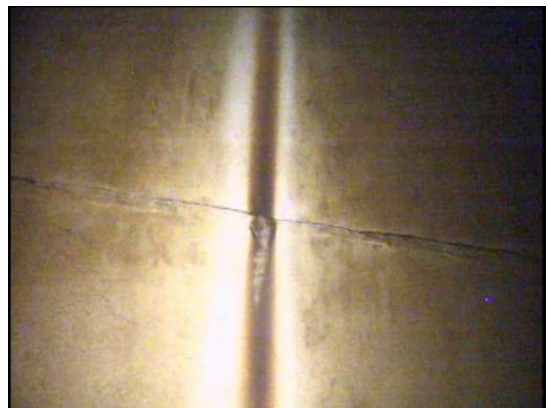
Shows an isolated area of rust and small tubercle formation on the shell surfaces below water
