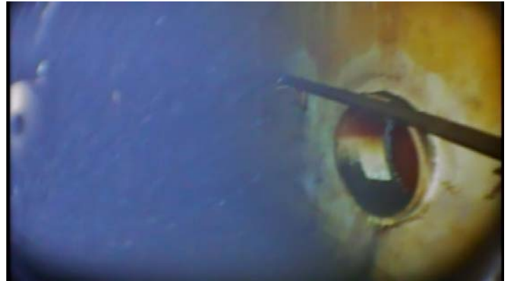
Showing the bubbler system along the interior of the bottom shell ring to be intact and in visually good condition
