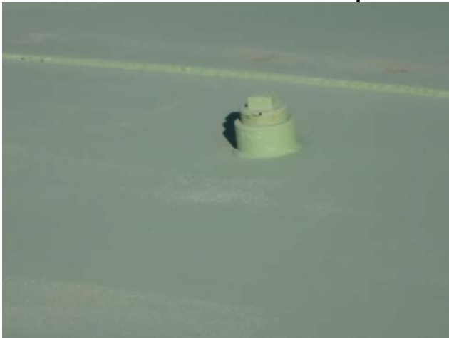
Showing roof rigging coupling to be intact, structurally sound and sealed by a threaded steel plug
