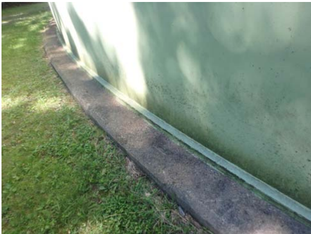
Showing junction between floor plate extension and foundation to be effectively sealed
