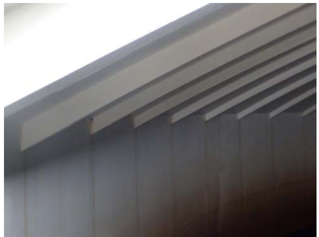
Showing only minor coating degradation and rusting along outer junction with shell and along rafter attachment points
