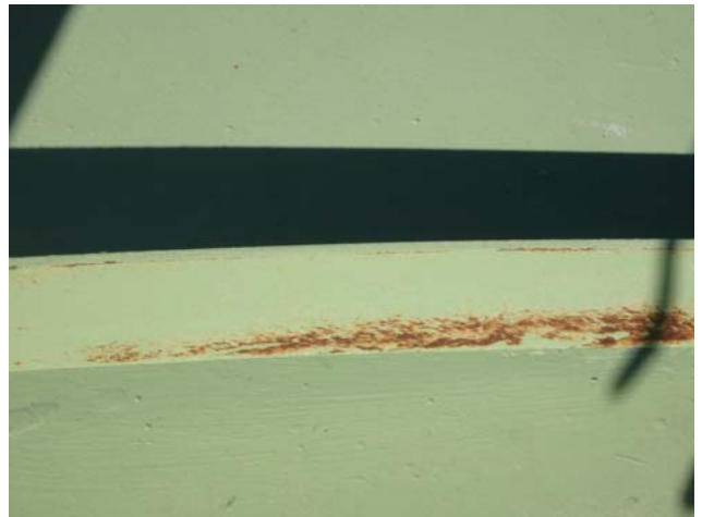
Showing localized area of coating degradation and rusting along toe plate of center handrail
