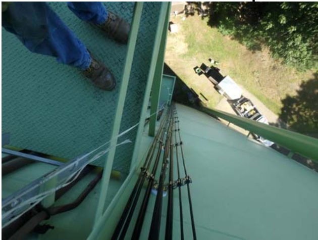
Showing run of antenna cables attached to the shell of the tank by magnetic mounts
