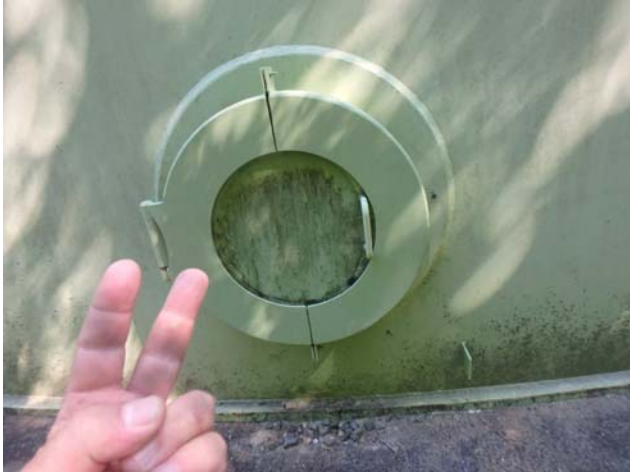
Showing the 2nd of (3) shell manholes all of which appear intact and structurally sound
