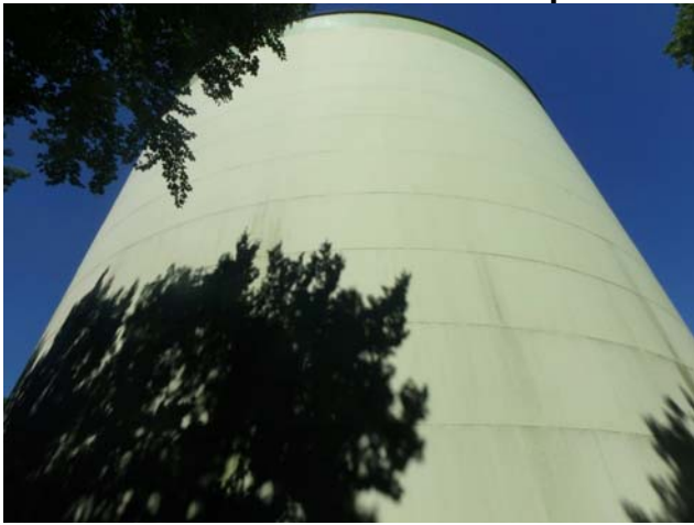
Coatings along the shell surfaces are in generally very good condition with minimal degradation evident
