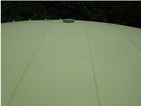
The exterior roof coating is weathered but exhibits little corrosion
