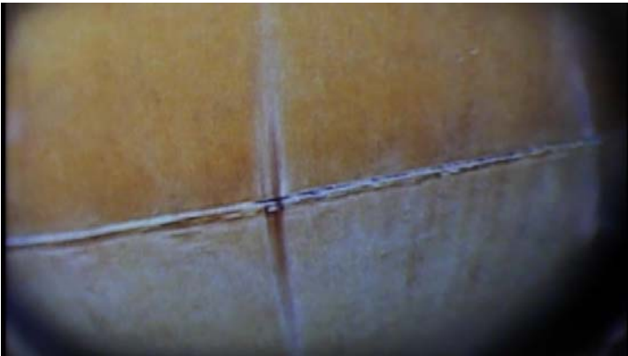
Showing isolated area of rust formation along interior horizontal weld seam
