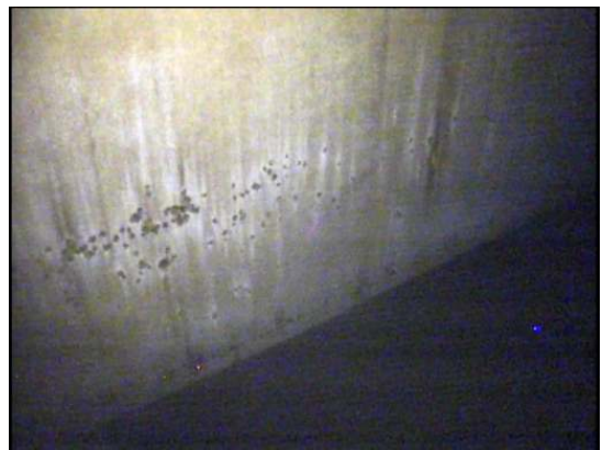
Shows areas of blistering and corrosion on the shell plates adjacent to the floor
