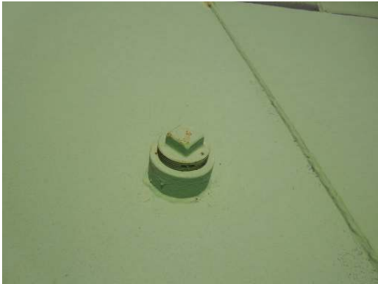
There is light rust located on the rigging coupling plugs
