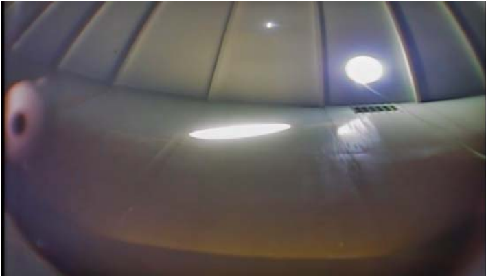
Coating along the upper shell surfaces appears to be in good condition with only heavy staining evident
