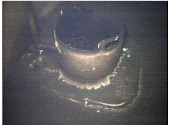
The coatings on the fill pipe silt trap and adjacent floor surfaces are stained
