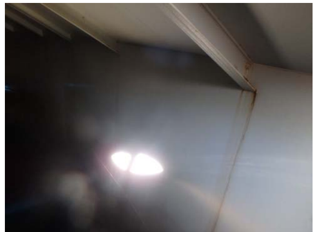
Showing evidence of localized rusting taking place where rafters attach to shell
