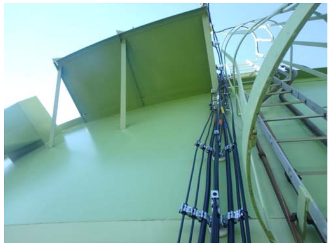
Showing run of antenna cables attached to the shell of the tank by magnetic mounts
