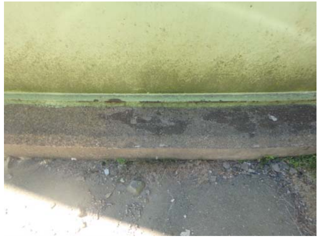
Showing minor degradation and rusting along floor plate extension
