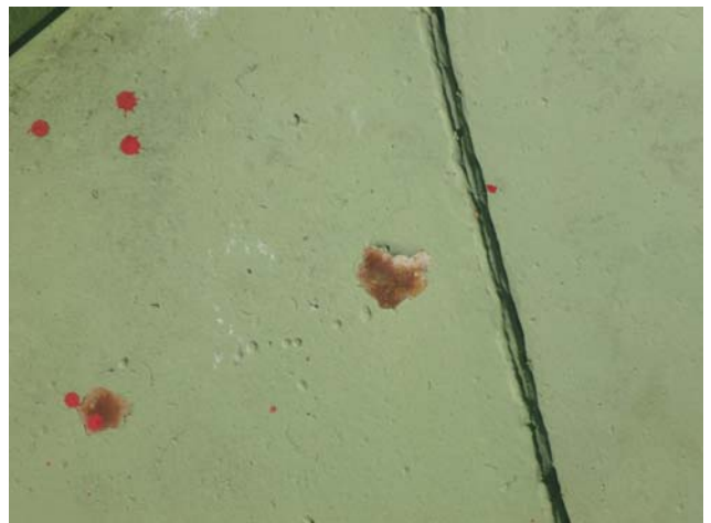
Showing additional areas of delaminated coating and rusting along the exterior of the roof
