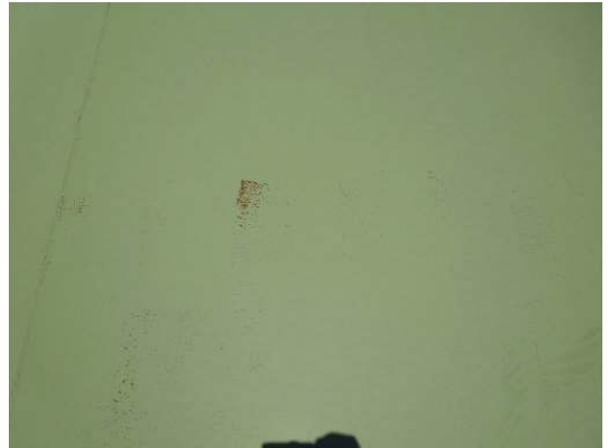
Shows scattered areas of exposed prime coat due to severe weathering of the top coats on the roof plates
