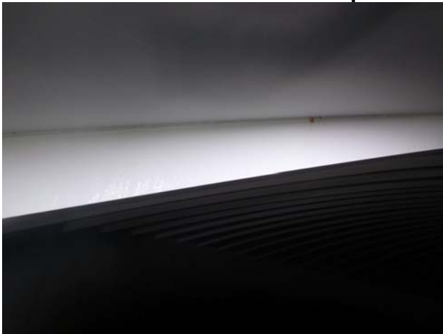
Showing evidence of very minor rusting along the underside of the roof
