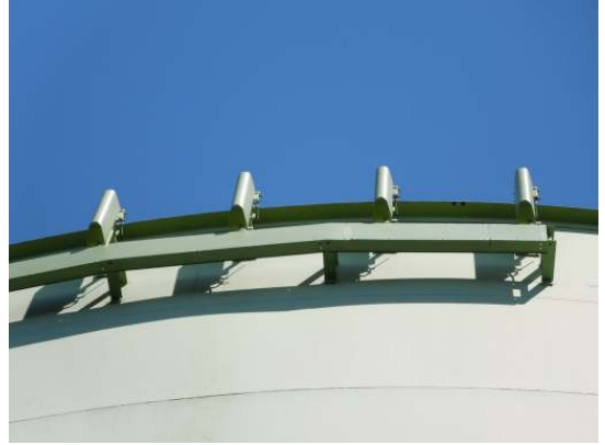
There is a series of cellular antennae and coax cable trays attached to the tank exterior
