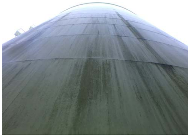
Coatings along the shell surfaces are in generally very good condition however heavily soiled
