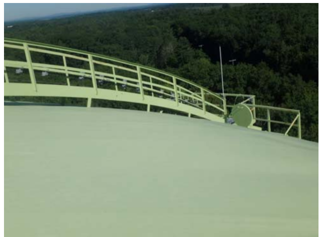
Showing coatings along the roof exterior surfaces to be in generally good condition
