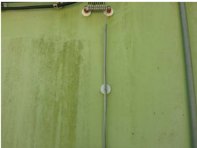
Showing ground wire magnetically mounted to the shell of the tank
