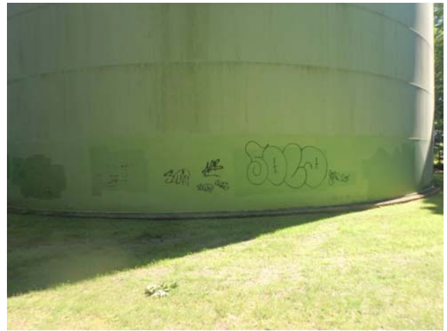
Showing additional painted graffiti applied to shell since last inspection
