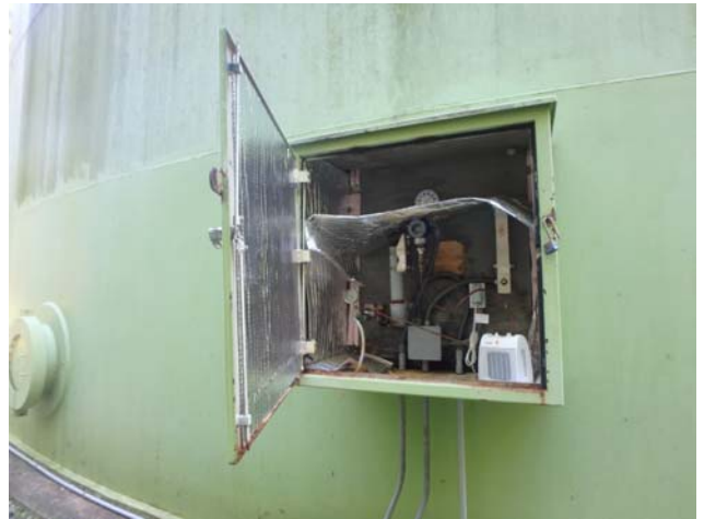
Showing telemetry box housing miscellaneous electrical and monitoring equipment
