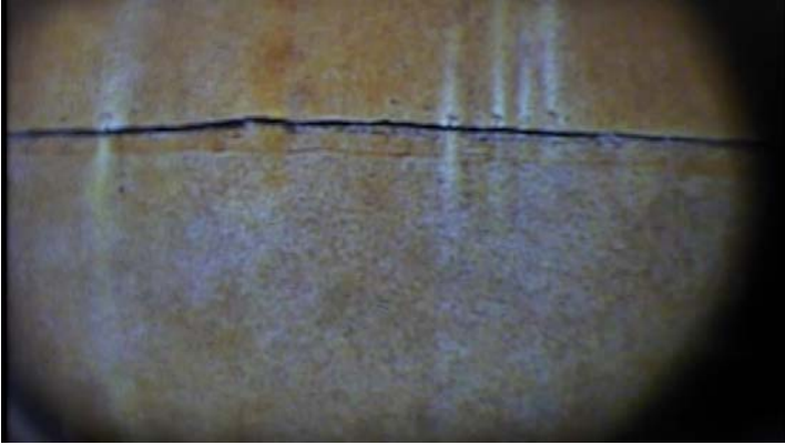
Showing isolated areas of small blisters along interior horizontal weld seam
