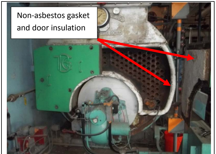
4. Front access doors in inactive boiler #3 with non-ACBM gaskets and door insulation.
