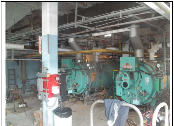
2. Overall boiler room with Cleaver Brooks Boilers.
