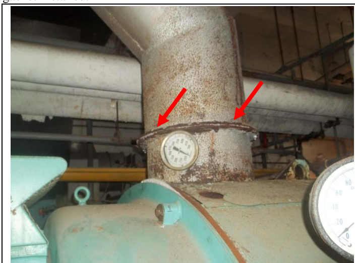
5. Exhaust duct above boilers with ACMG gasket at flanges (arrow).
