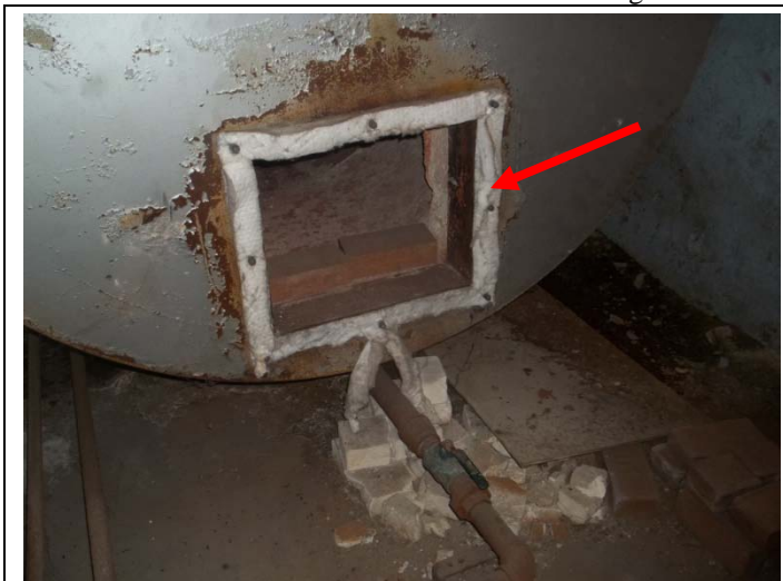
3. Cleanout door in rear of inactive boiler #3 with non-asbestos gasket installed.
