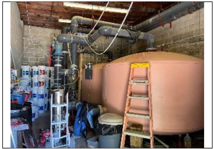
8. Interior view of the Pump House.
