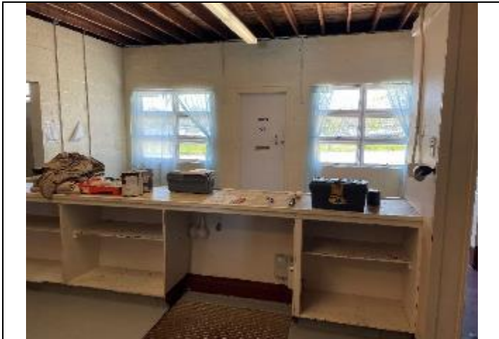
3. View of the lobby from behind the snack bar in the Bath House. ACBM patching material is located on the wall entering the women's changing area.
