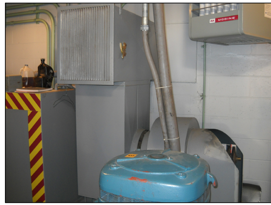
EXISTING DRY WELL FAN AND DUCTING
