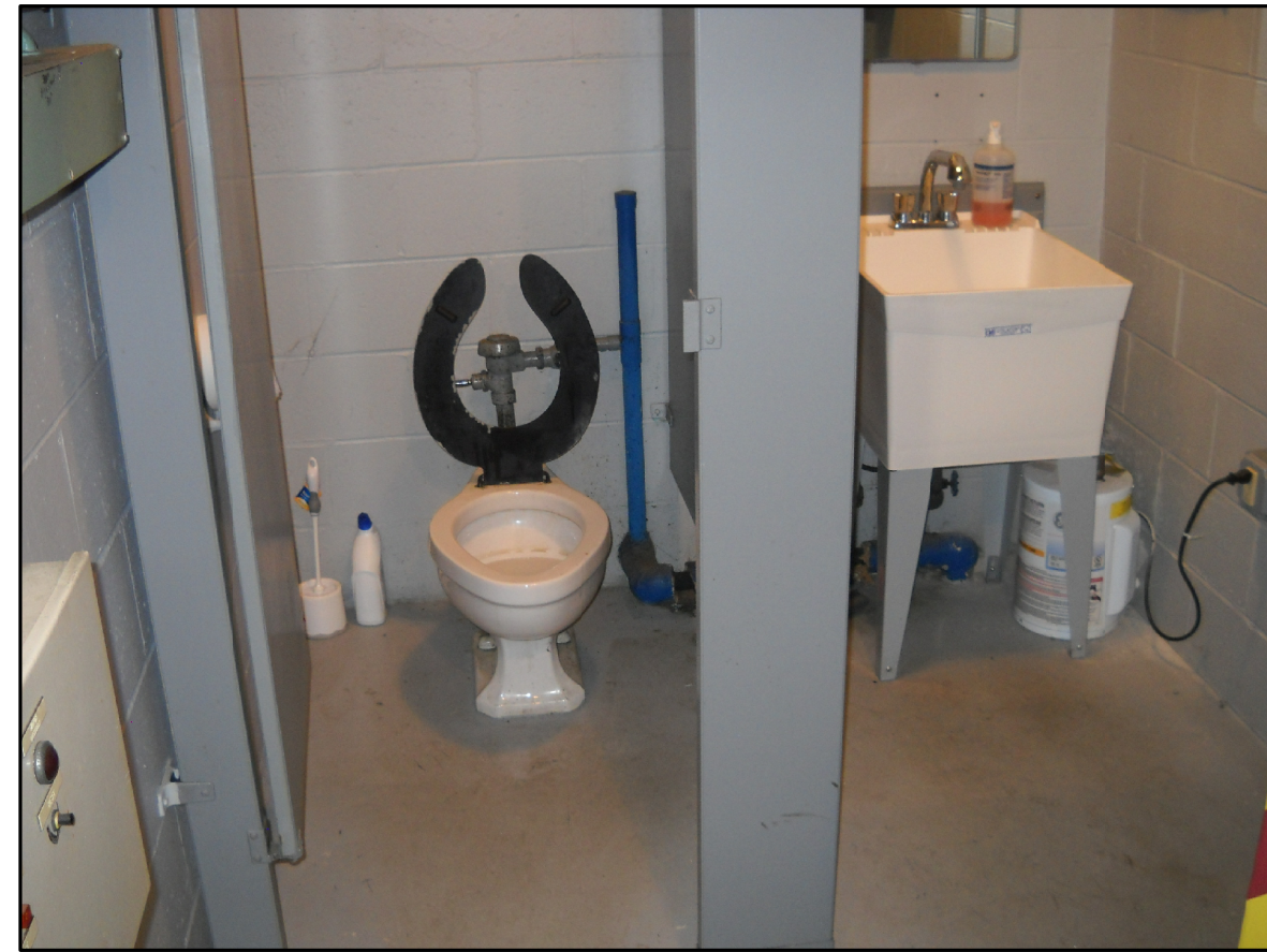
EXISTING WATER CLOSET, SINK, AND HOT WATER HEATER.
