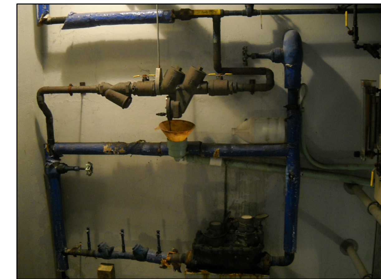
EXISTING WATER SERVICE ENTRANCE.
