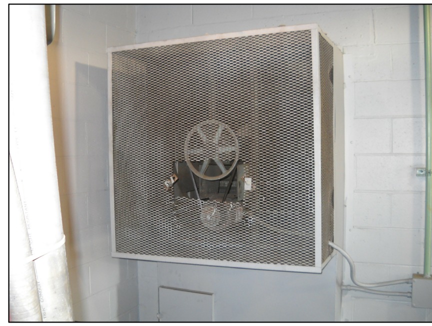
EXISTING DRY WELL EXHAUST FAN
