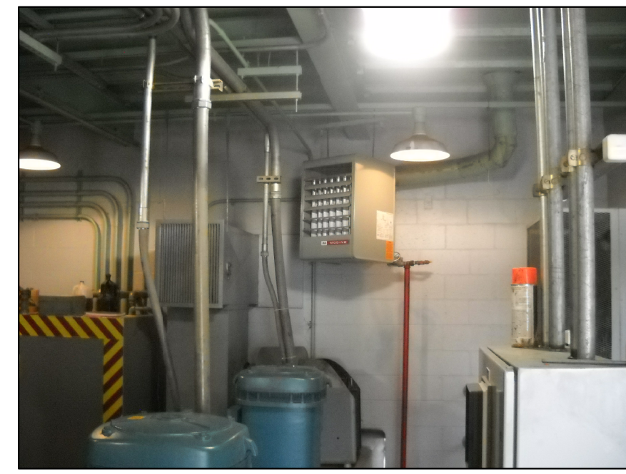
EXISTING UNIT HEATER AND EXHAUST DUCTING
