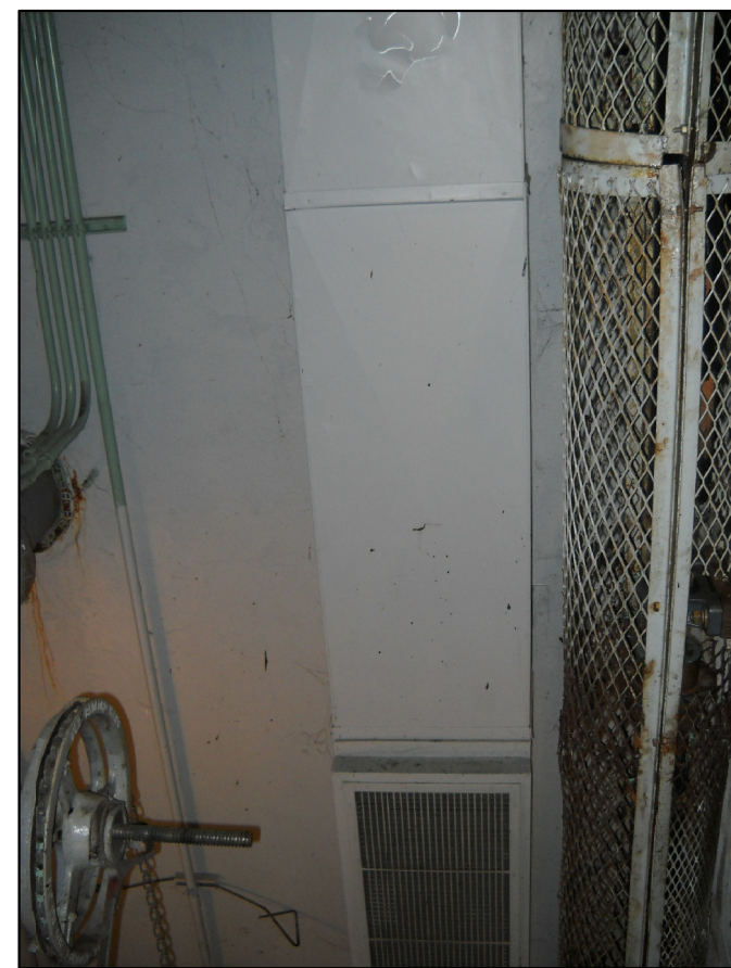
DRY WELL DUCTING
