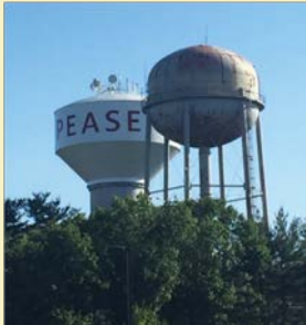
Water Storage Tank
