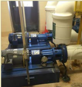
Grafton Road Water Facility Booster Pumps
