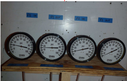
Gages to monitor pressure into and out of Filters 1 & 2
